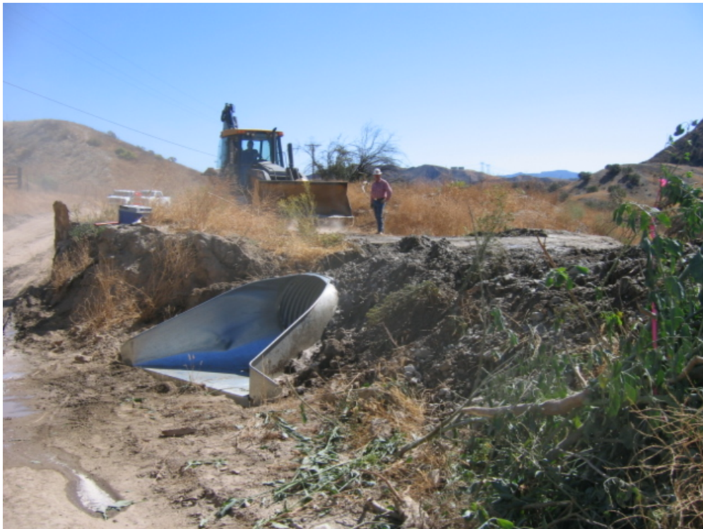
Figure 2: A collapsed culvert was replaced along the access road approaching NC 27, Section 1.
