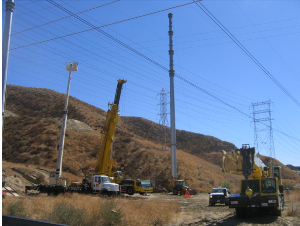
Figure 1: Steel poles and crane guard structures being erected at Haskell Canyon for the LADWP utility crossing.
