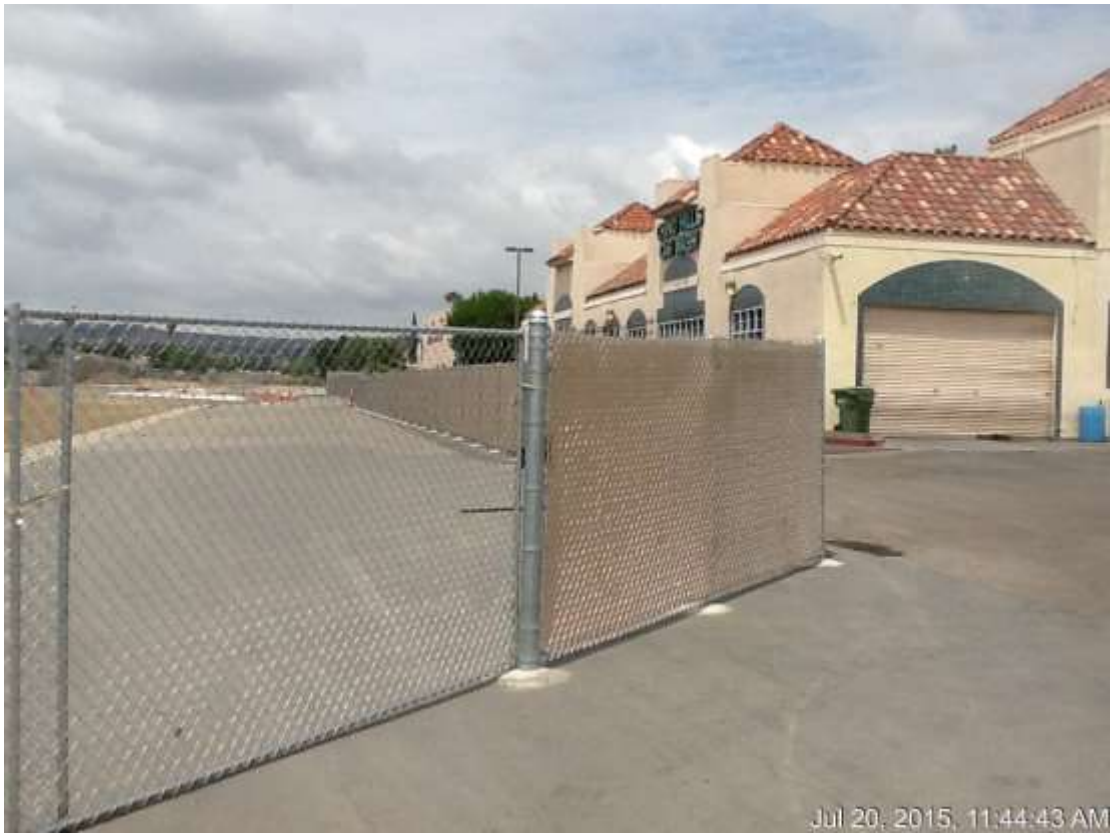
Figure 3: Fence installation at VC #14 along the shopping center Fire Lane, 500 kV Underground.
