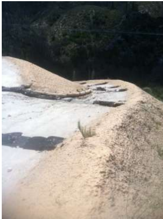
Figure 3: Erosion evident at Construct 68, Segment 6B. BMPs were scheduled for maintenance during the reporting week.
