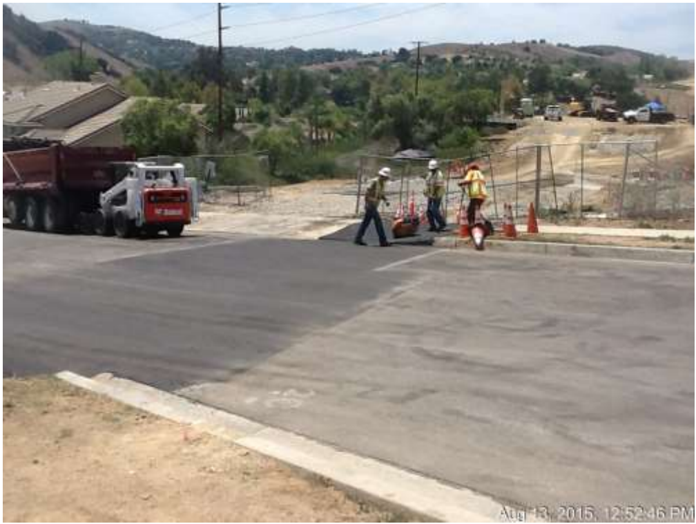
Figure 3: Temporary sidewalk installation along the trench line on Maplewood Drive, 500 kV Underground.
