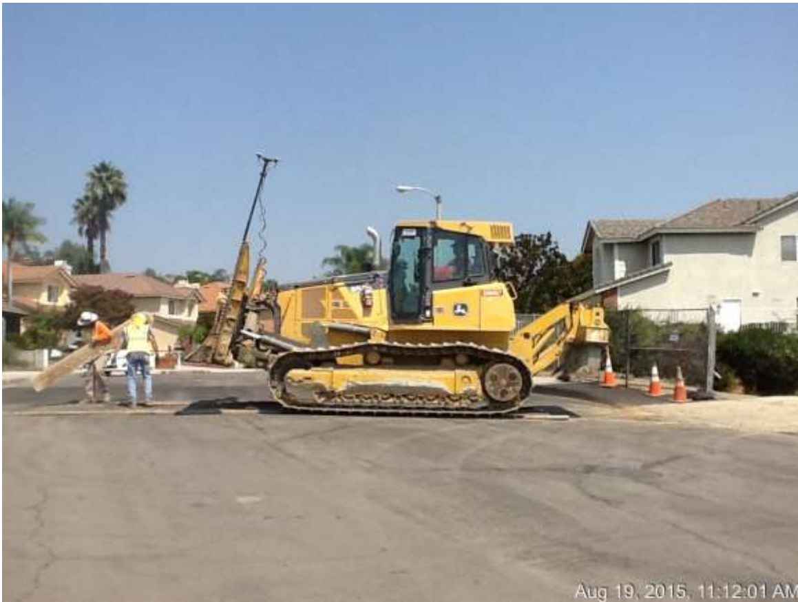
Figure 7: Equipment crossing Morningfield Drive without traffic control in place, 500 kV Underground.
