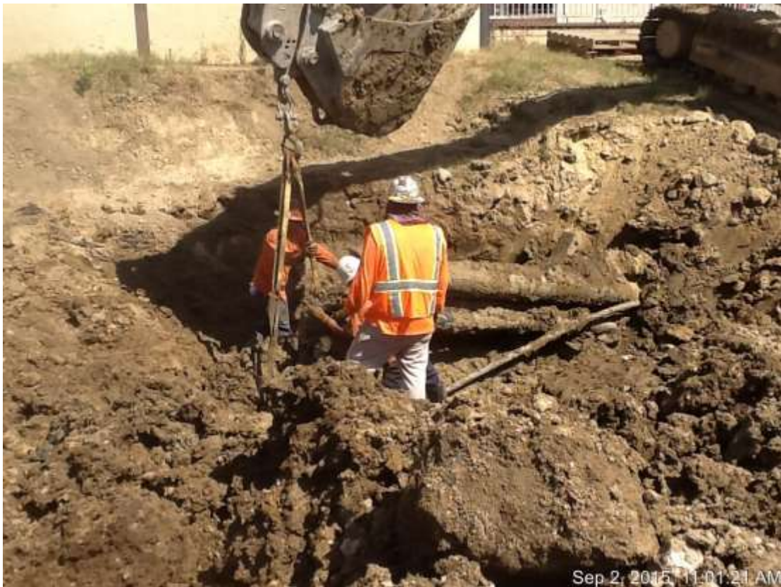
Figure 6: Conduit being excavated at VC #11 after successful pull of HDD C1-S2, 500 kV Underground.
