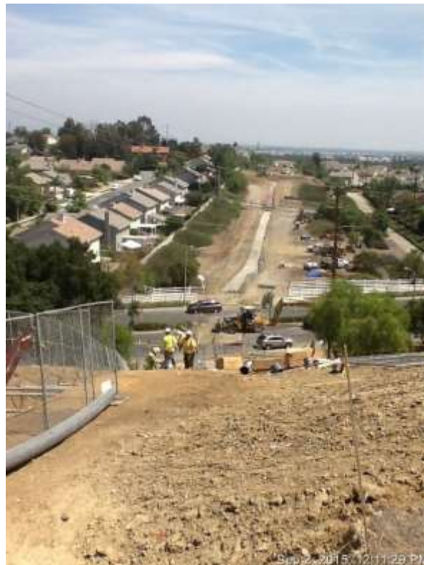
Figure 2: Conduit placement in trenchline between VC #8 and Chino Hills Parkway, 500 kV Underground.
