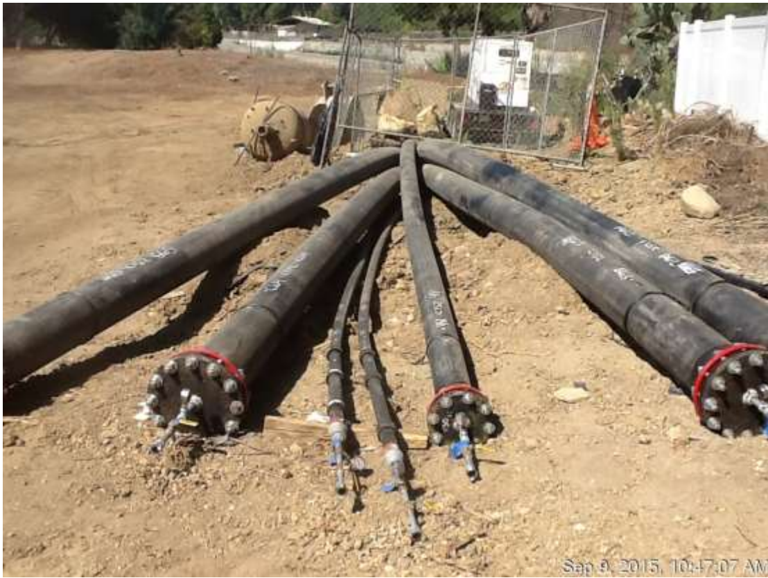
Figure 5: Conduit ends for completed conduit pull at long bore HDD C1-S2, 500 kV Underground.
