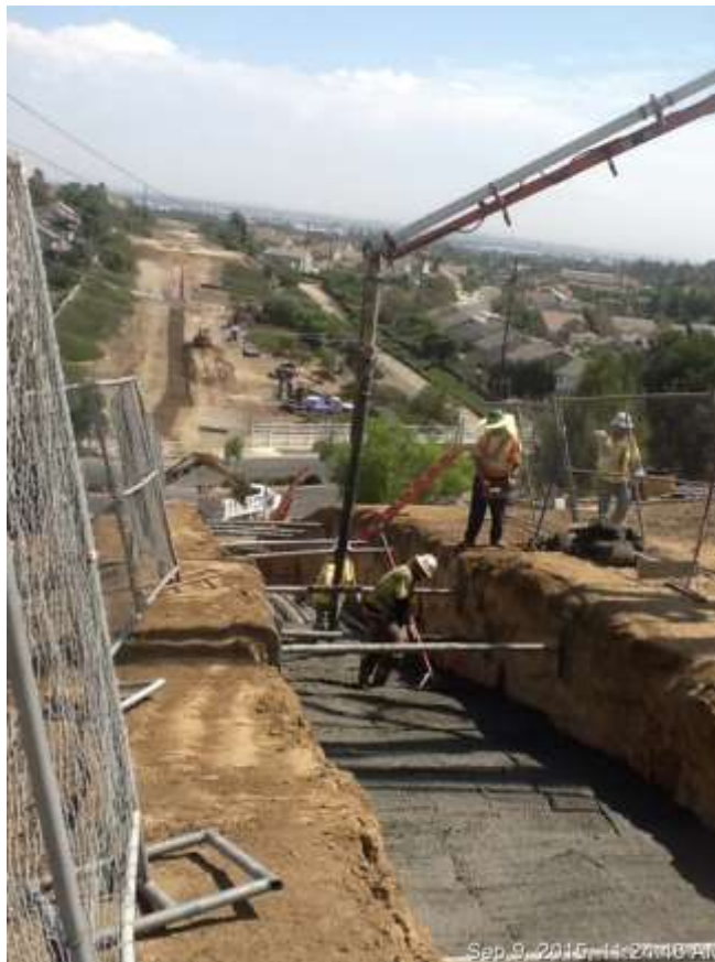
Figure 3: Concrete pouring activities within conduit trench between VC #8 and Chino Hills Parkway, 500 kV Underground.
