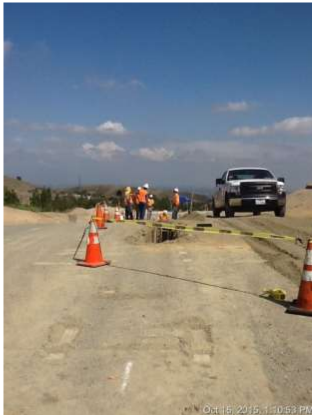
Figure 2: Telecom installation between VC #1 and WTS, 500 kV Underground.
