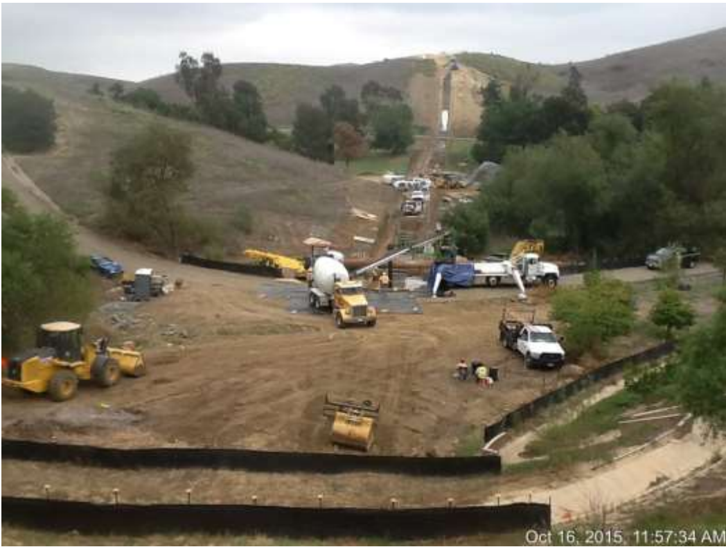
Figure 3: Conduit backfill at stream diversion between VC #2 and Canon Lane, 500 kV Underground.
