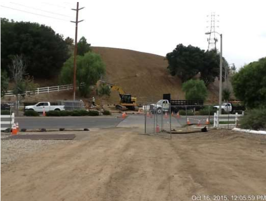
Figure 4: Grading activities on slope between Chino Hills Parkway and VC #8, 500 kV Underground.
