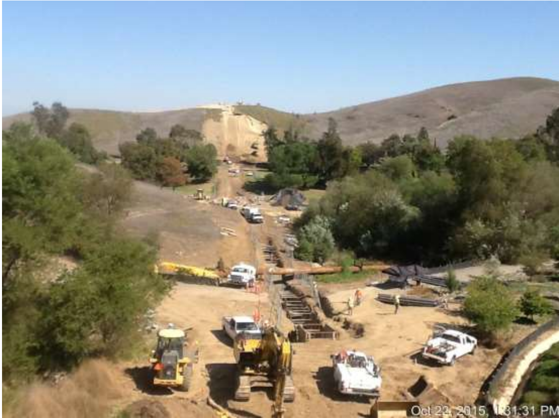
Figure 1: Conduit trenching under the stream diversion between VC #2 and VC #3, 500 kV Underground.
