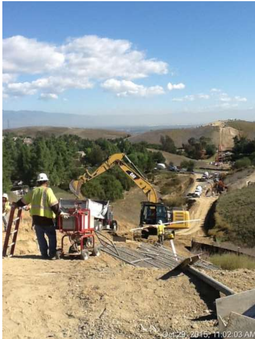
Figure 2: Trenching operations near VC #1 looking east toward Canon Lane and golf course, Chino Hills, 500 kV Underground.
