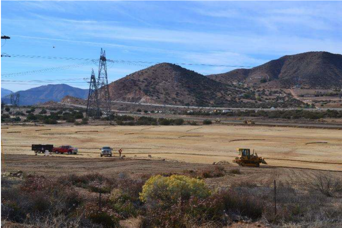
Figure 1: Decompanction work was conducted in preparation for hydroseeding at South Vincent Yard, Segment 11C.
