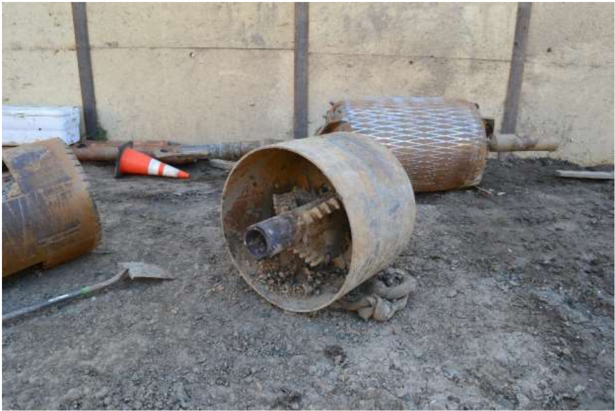
Figure 3: The basket drum which had been stuck in HDD Bore Location 2 hole was retrieved over the weekend, 500 kV Underground.
