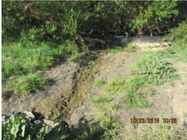
Figure 1: Erosion repairs were identified at a discharge point at the WTS in October, the repairs are pending the issuance of wetland permit amendments, photo courtesy of FRED.
