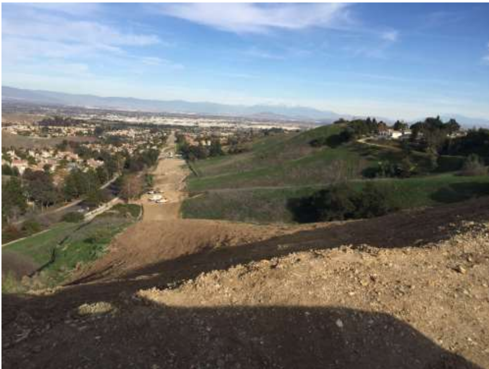
Figure 2: Restoration grading operations from VC #4 (at the bottom of the hill) to VC #3. Permanent BMPs are installed as crews complete the grading, then the area is treated with hydroseed.
