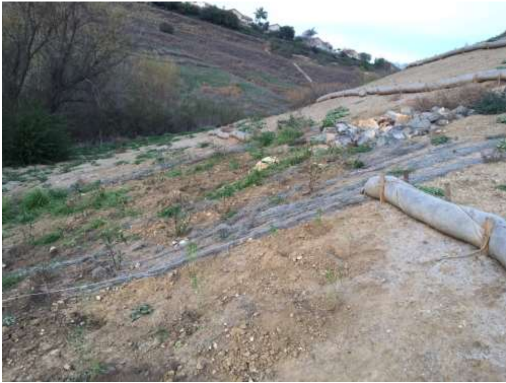
Figure 5: Container plants installed at the wrong location downslope from the WTS. SCE has indicated that rather than removing the plants and moving them, additional plants would be purchased and installed in the correct location.
