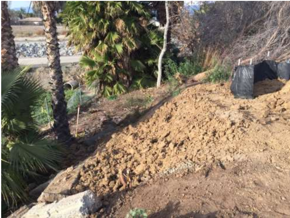
Figure 6: Freshly disturbed soils without downslope BMPs near VC #12. This location drains to the Chino Creek flood control channel. BMPs were later installed at this location.
