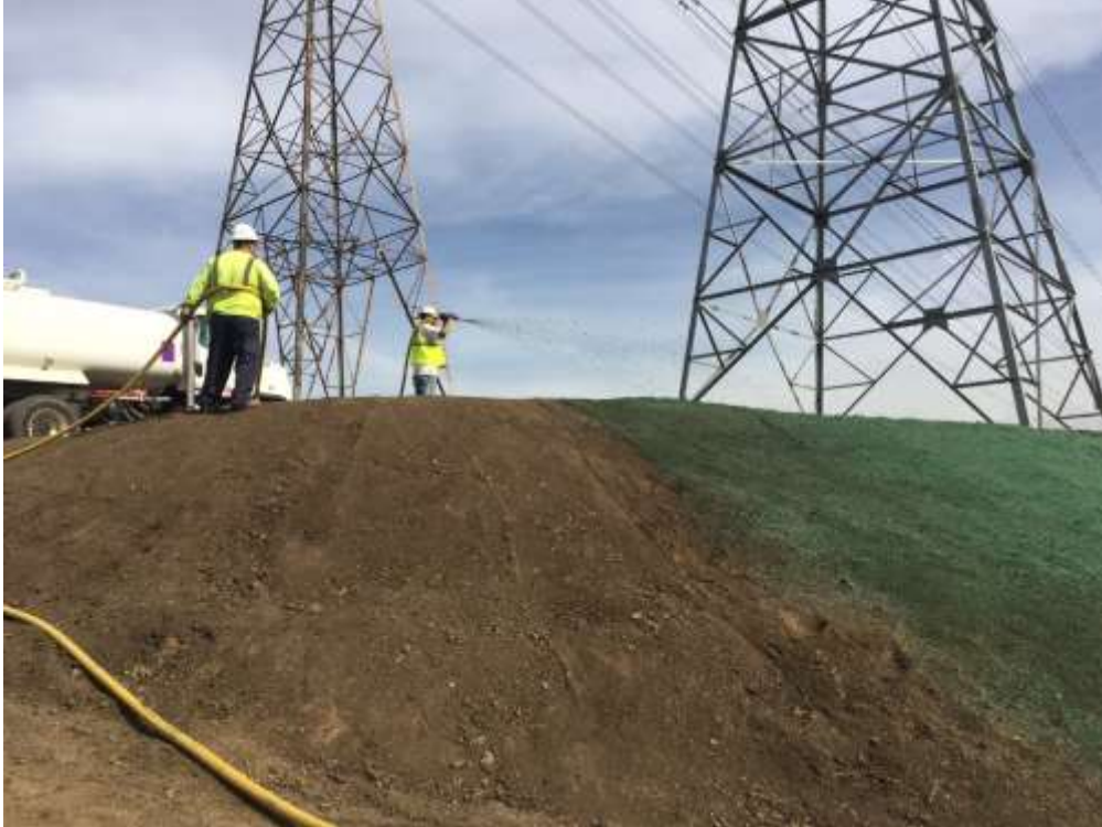
Figure 1: Restoration crews spraying hydroseed in Segment 8 Phase 4. Prior to hydroseed application, the sites are weeded.
