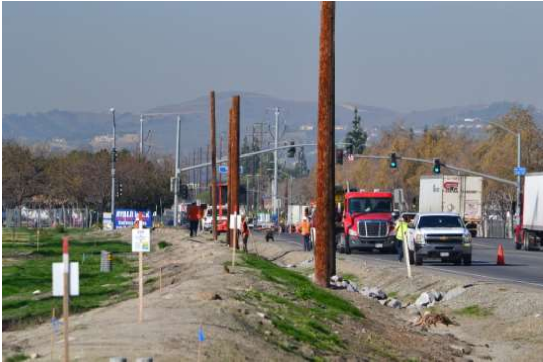
Figure 1: 66 kV crews conducting telecom pole removal along Edison Avenue in the City of Chino.
