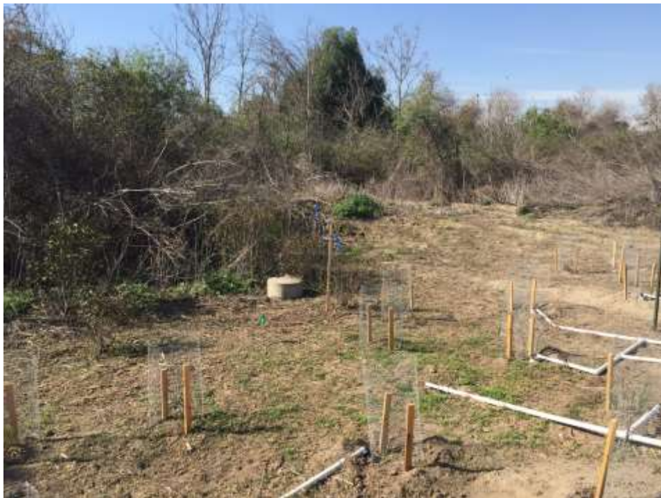
Figure 2: Henkels and McCoy crews mobilized to Whittier Narrows Tower M41-T5 to removed four foundations left by a previous contractor. Recently planted container plants had to be removed in order for equipment to access the foundations.
