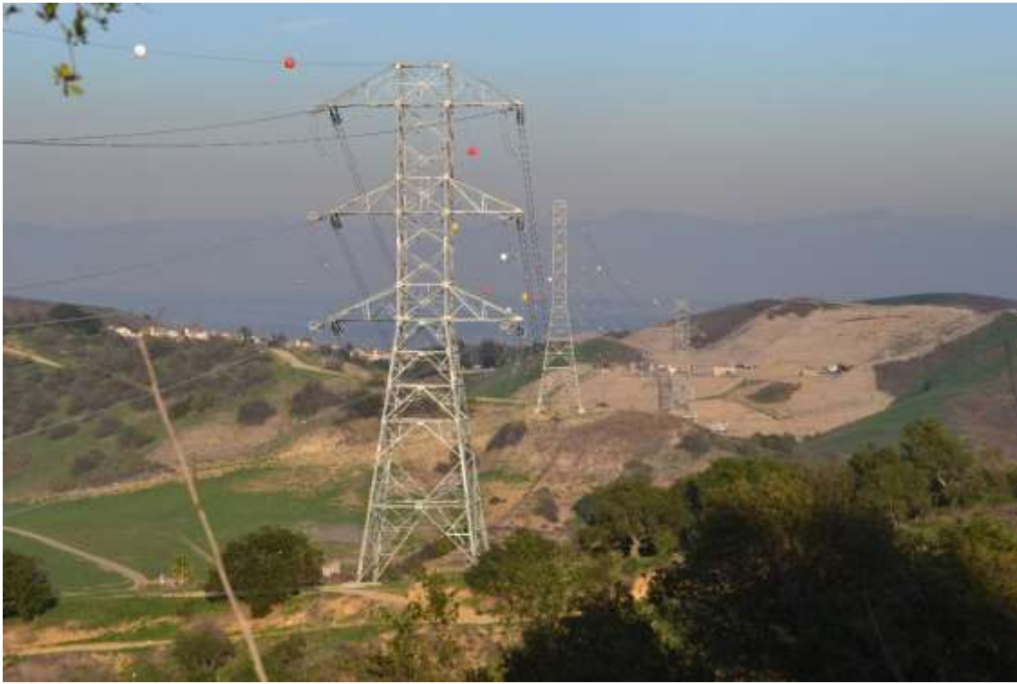
Figure 3: Conductor installation including marker ball installation was completed to Tower M60-T1 near the WTS, 500 kV Underground.
