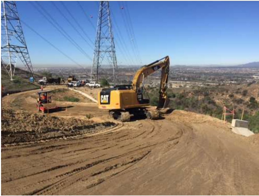
Figure 2: Crews mobilized to Tower M43-T3 on Segment 8 to conduct civil repairs to the access road and to expand the rip rap area for offsite sediment control.
