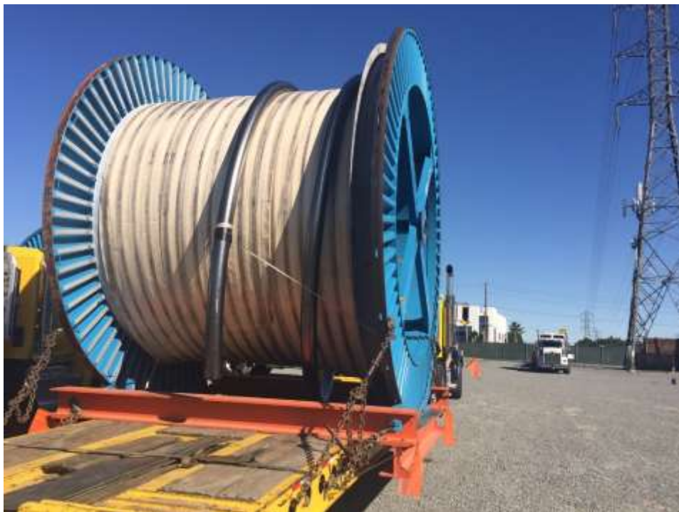
Figure 6: Cable reels stored at the Mira Loma yard and delivered to the right-of-way, 500 kV Underground.
