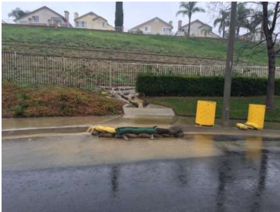
Figure 5: Runoff from project right-of way onto public streets, 500 kV Underground.
