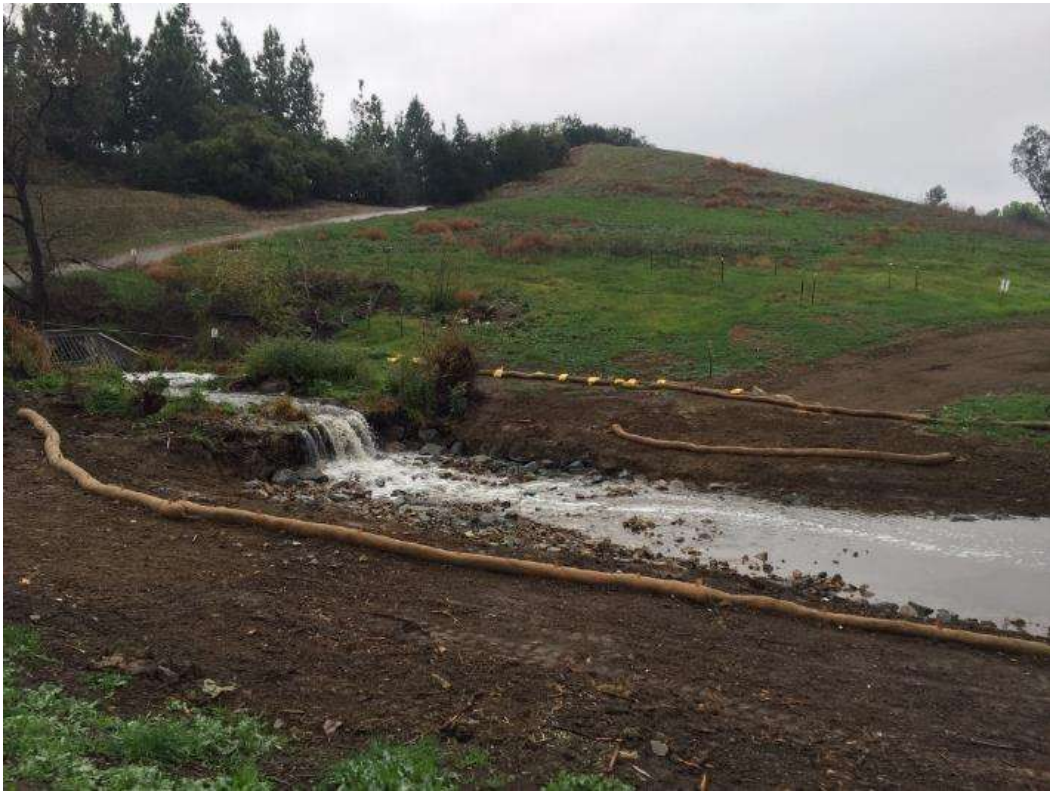
Figure 2: Site of stream diversion near VC #2 after diversion materials have been removed, 500 kV Underground.
