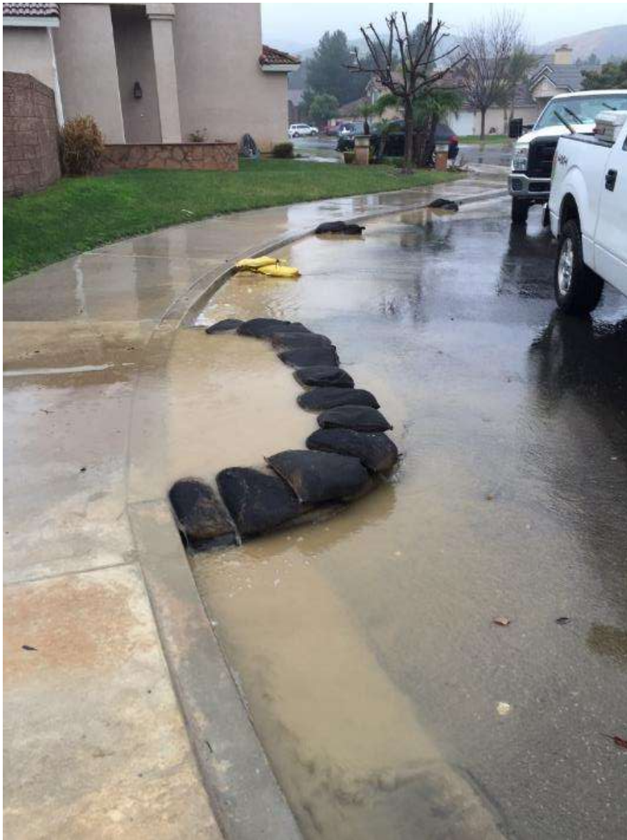
Figure 7: Runoff from project right-of way onto public streets, 500 kV Underground.
