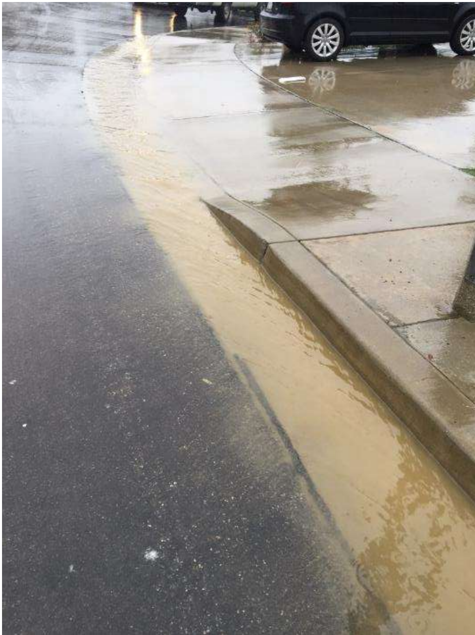
Figure 6: Runoff from project right-of way onto public streets, 500 kV Underground.
