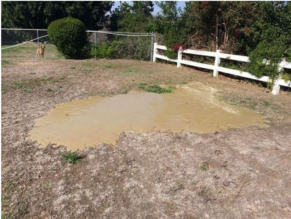
Figure 6: Frac-out on private property near VC #12, 500 kV Underground (Photo courtesy of SCE).
