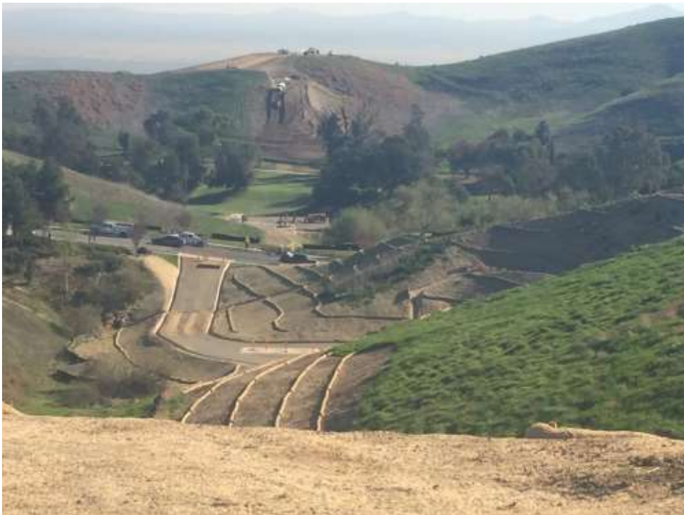
Figure 2: Restoration grading and permanent BMP installation between VC #1 and VC #3, 500 kV Underground.
