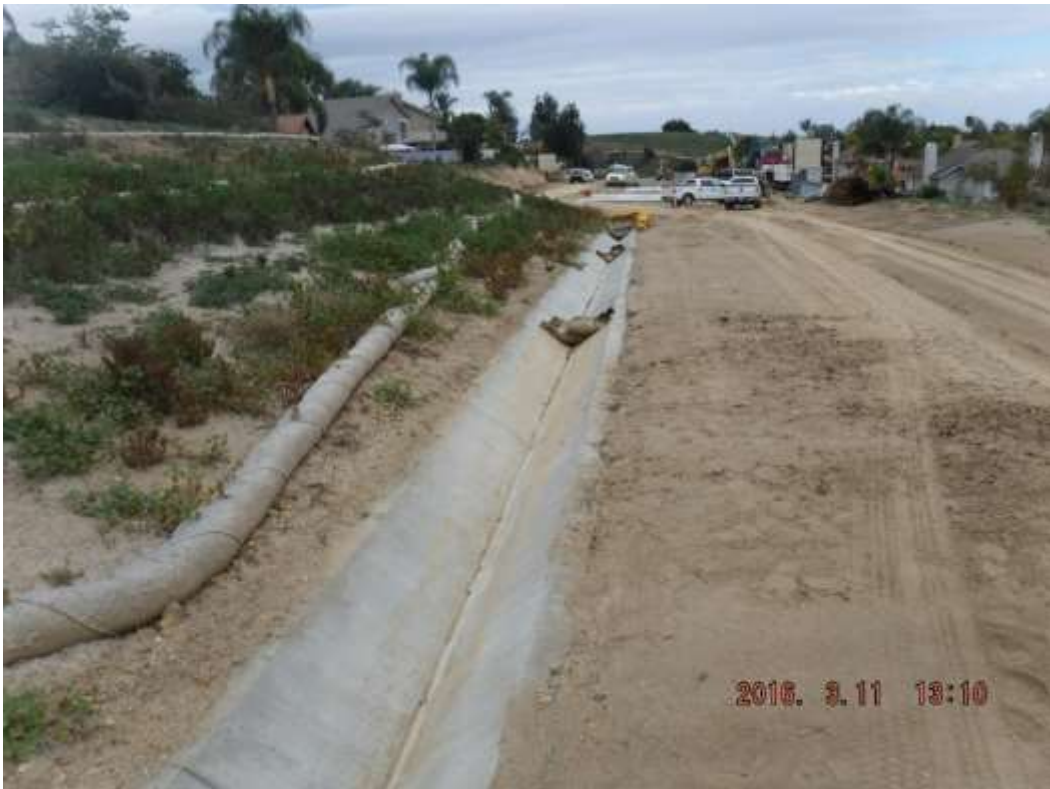
Figure 6: After cleanup of sediment in v-ditch between VC #10 and #11, 500 kV Underground. (Photo courtesy of SCE)
