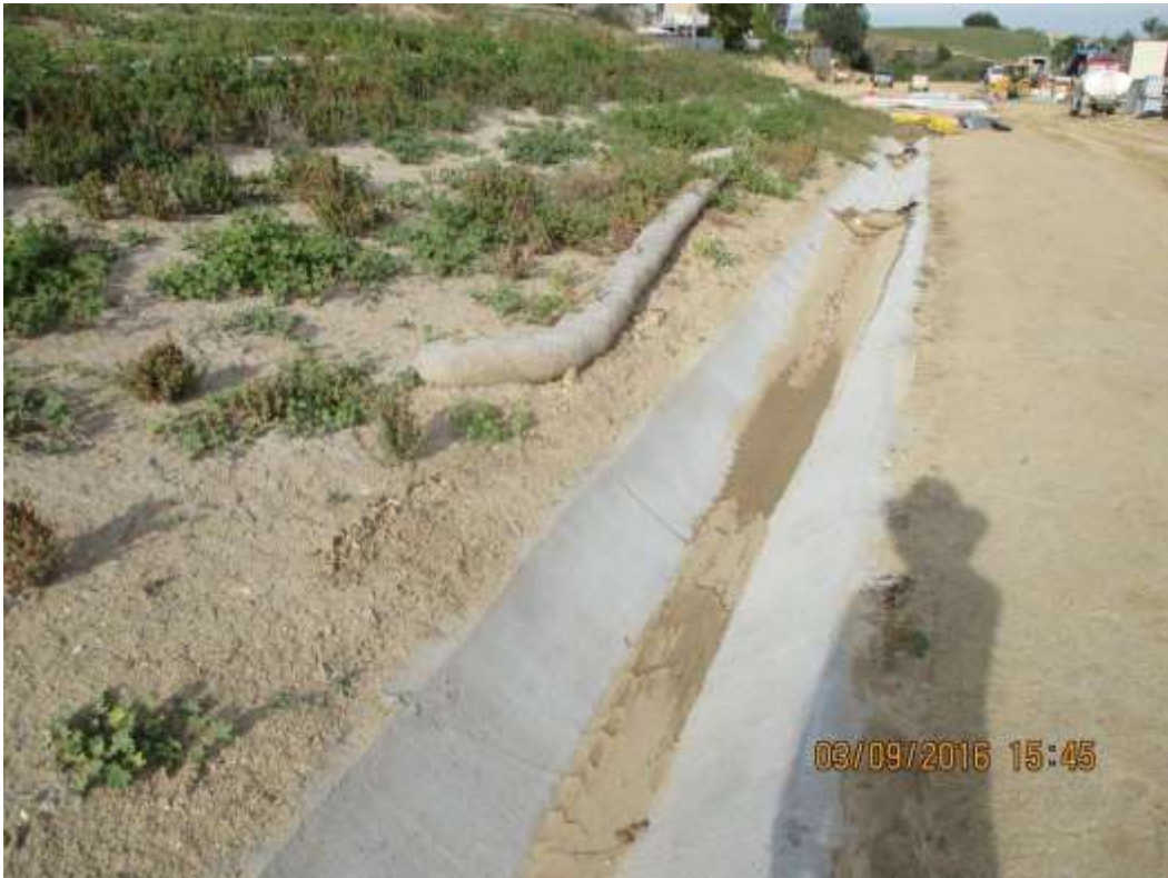
Figure 5: Sediment in concrete v-ditch between VC #10 and #11. (Photo courtesy of SCE)
