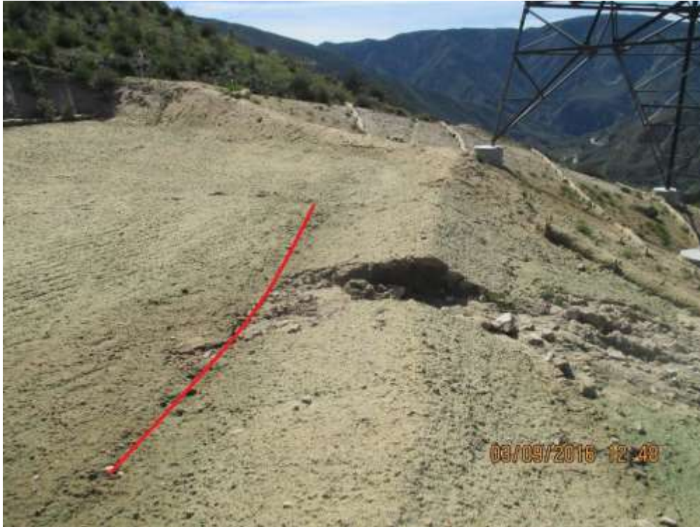
Figure 1: Erosion off of recently restored and decompacted area at Tower 54, Segment 11C. (Photo courtesy of SCE)
