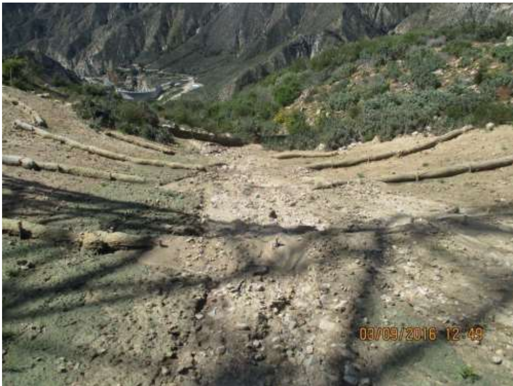
Figure 2: Erosion off of recently restored and decompacted area at Tower 54, Segment 11C. (Photo courtesy of SCE)
