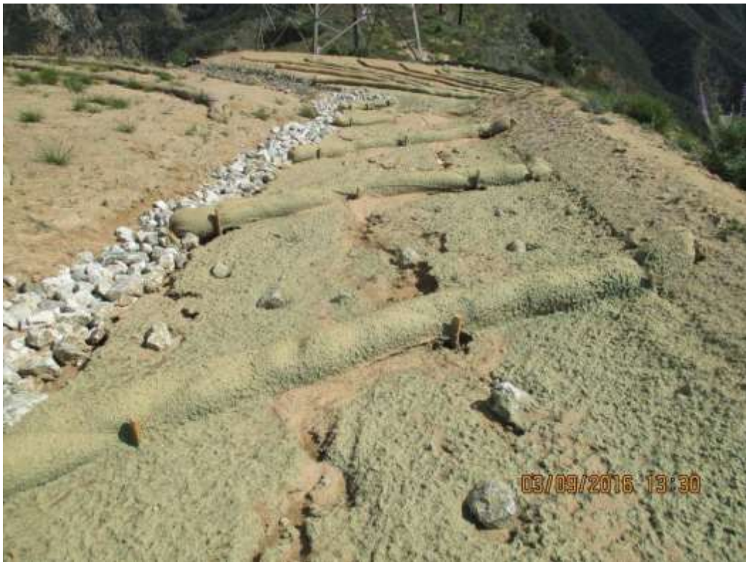
Figure 3: Erosion off of recently restored and decompacted area at Tower 63, Segment 11C. (Photo courtesy of SCE)
