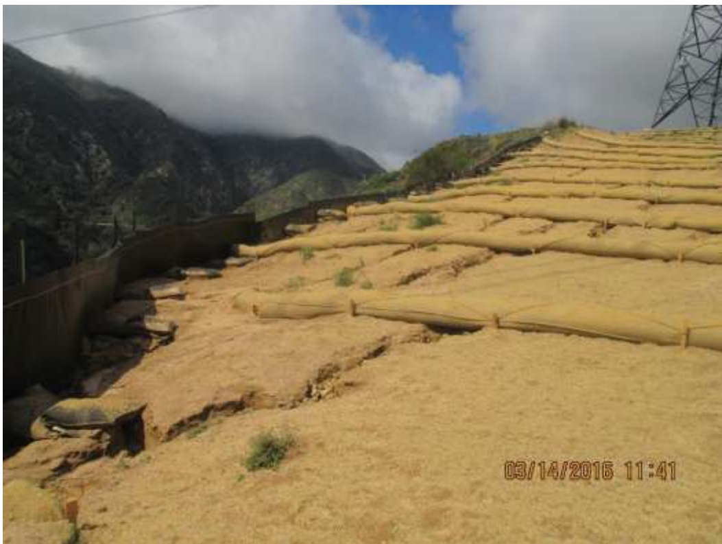
Figure 4: Erosion off of recently restored and decompacted area at Tower 54, Segment 11C. (Photo courtesy of SCE)
