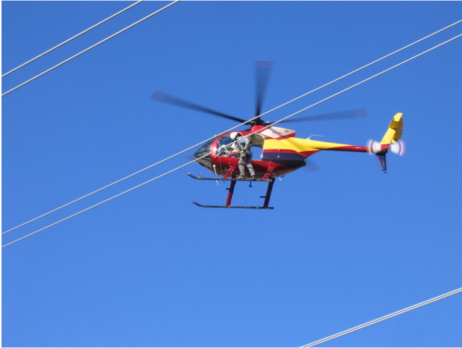
Figure 1: A helicopter was used to install spacers between the subconductors in Section 1.
