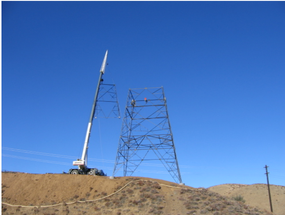
Figure 4: On Section 3, crews continue to construct the new single circuit towers near the Antelope Substation.
