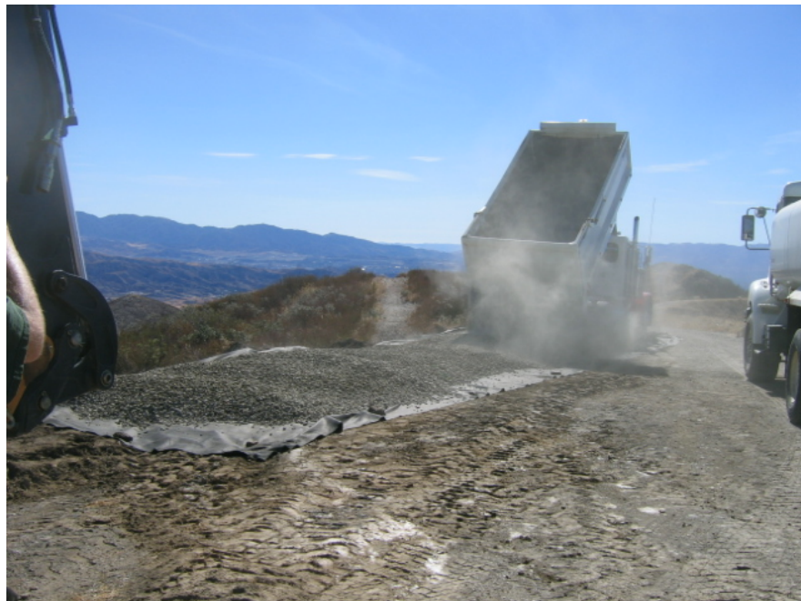
Figure 2: The installation of a wheel wash station at the start of access road SR-41 on the ANF, Section 2.
