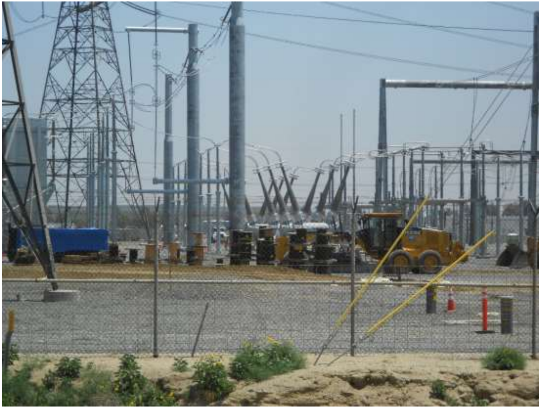
Figure 5: Ongoing work at the Mira Loma Substation associated with the 500 kV Underground work. Photo courtesy of SCE.
