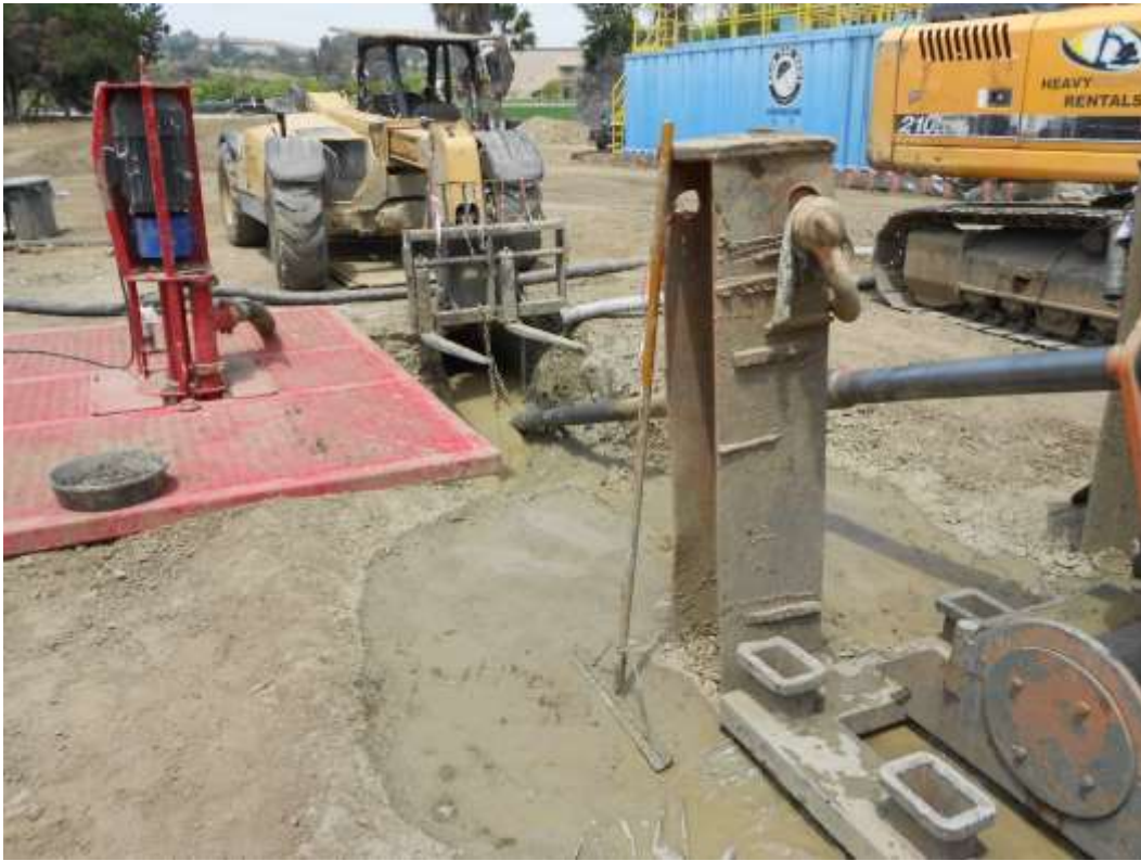
Figure 3: HDD operations near VC #12, entry pit of reaming operation, 500 kV Underground. Photo courtesy of SCE.
