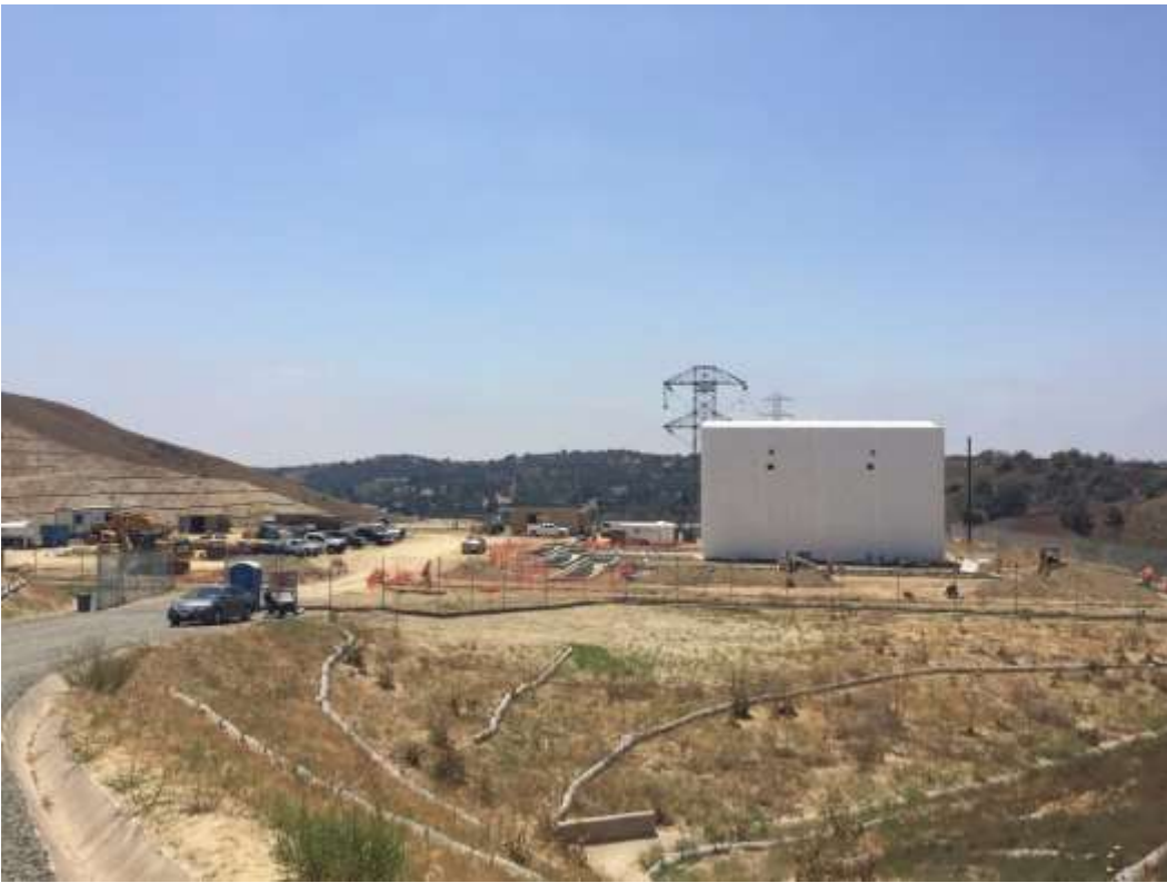
Figure 4: Construction including cable splicing and telecom conduit excavation continues at the WTS, 500 kV Underground.
