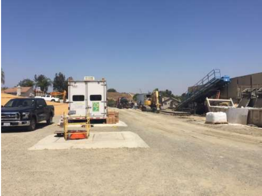
Figure 1: HDD reaming continues near VC #11 and cable splicing occurred at VC #11, 500 kV Underground.
