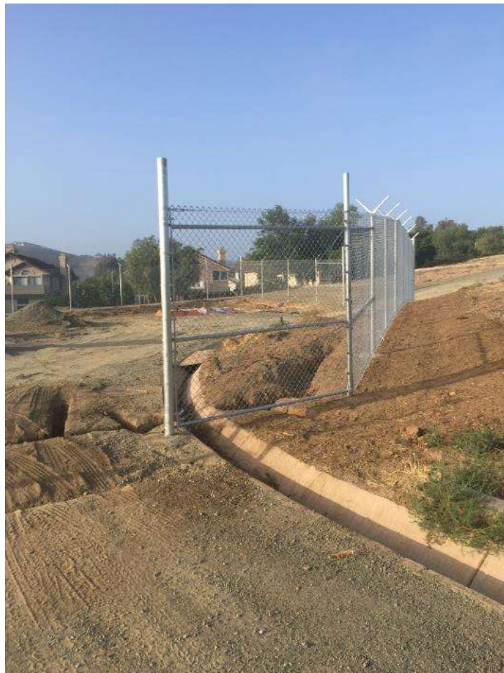
Figure 7: Fencing and uncapped fence post at VC #8, 500 kV Underground.
