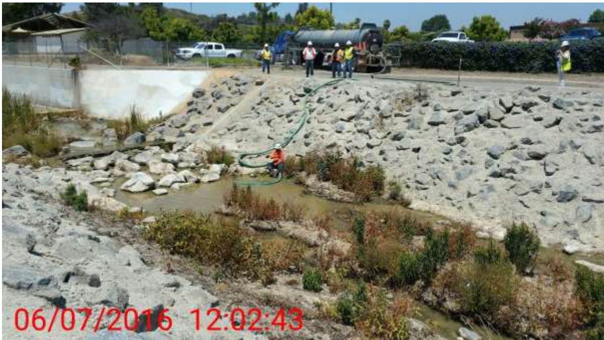
Figure 4: Vacuum trucks were mobilized to remove the silty water from the Carbon Canyon Creek, 500 kV Underground. Photo courtesy of SCE.
