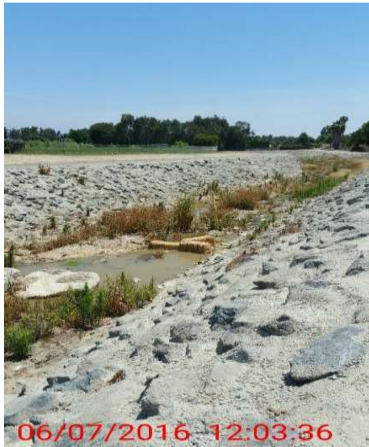
Figure 3: Hay bales were installed to help contain the sediment laden water that was discharged into Carbon Canyon Creek, 500 kV Underground. Photo courtesy of SCE.
