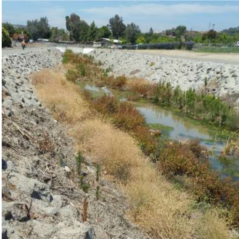
Figure 1: HDD construction was halted on June 7 after crews observed sediment laden water in the Carbon Canyon Creek, 500 kV Underground. Photo courtesy of SCE.
