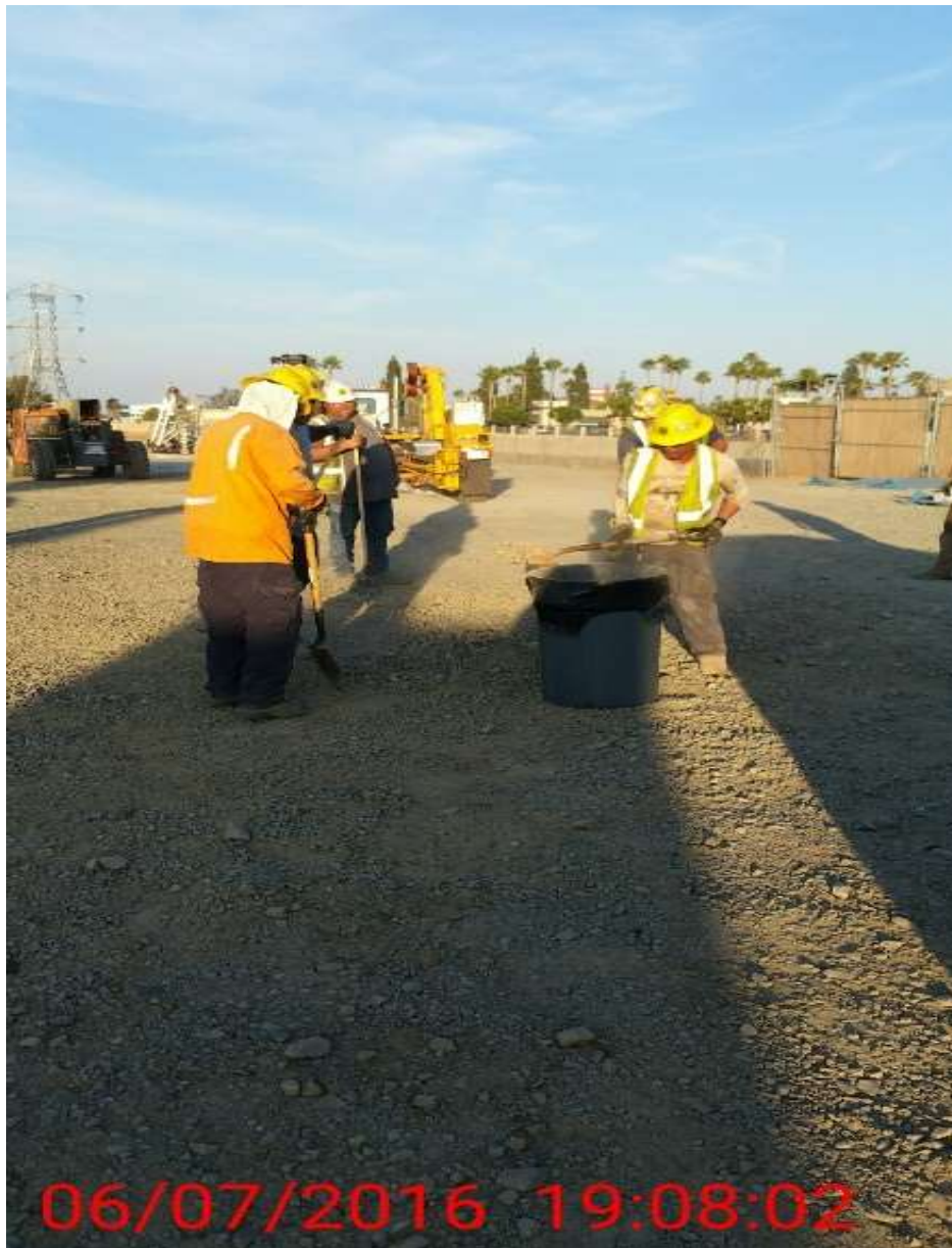
Figure 5: Spill from hydraulic leak near VC #14, 500 kV Underground. (Photo courtesy of SCE.)
