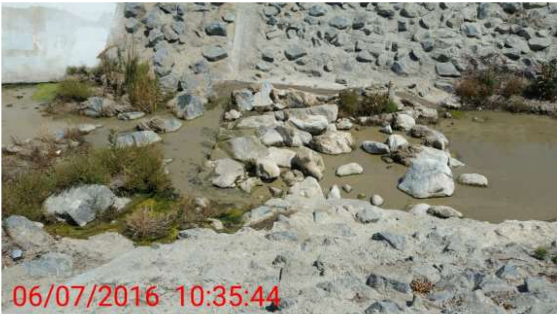
Figure 2: HDD Construction was halted on June 7 after crews observed sediment laden water in the Carbon Canyon Creek, 500 kV Underground. Photo courtesy of SCE.
