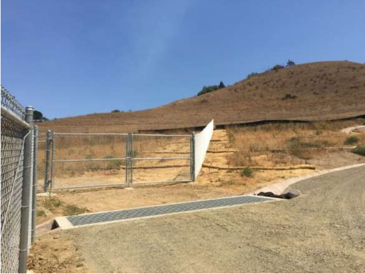
Figure 1: Temporary fencing was installed between Hope for the Hills Park and Restraint Vault #4, 500 kV Underground.
