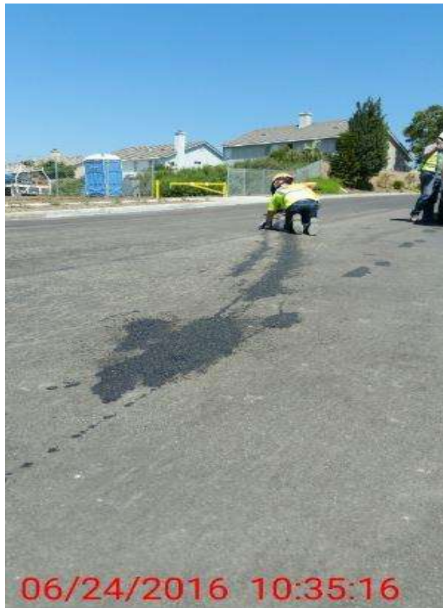
Figure 6: Spill clean-up, 500 kV Underground. (Photo courtesy of SCE)
