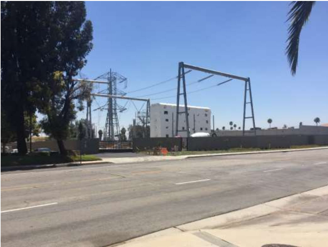
Figure 3: Work at the ETS included dismantling of the scaffolding for the cable terminations, 500 kV Underground.
