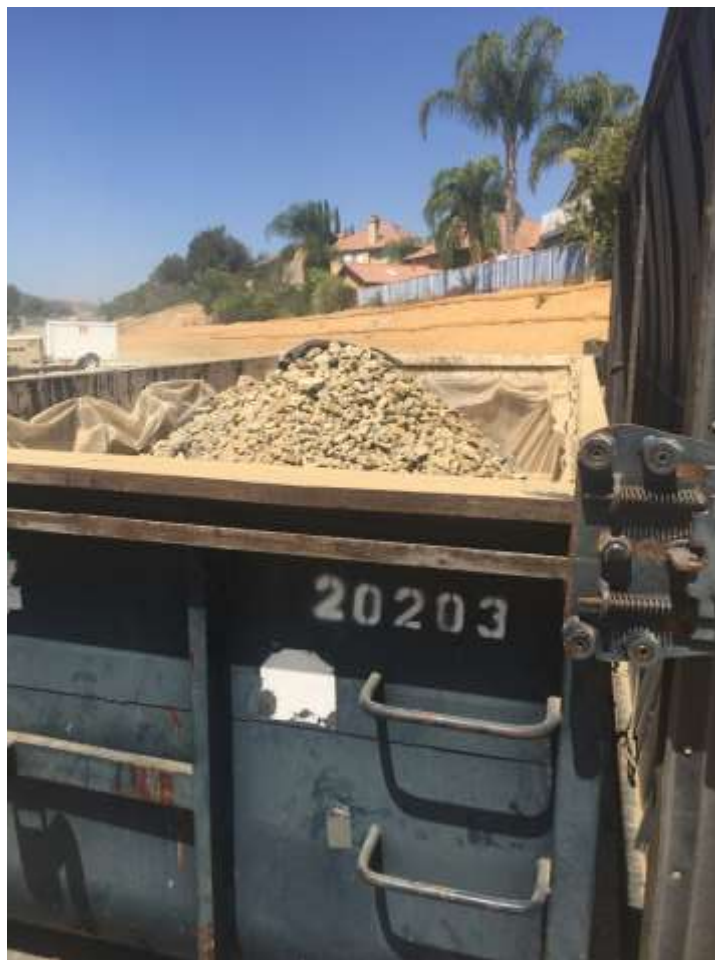
Figure 6: Contaminated material from hydraulic spill at VC #11 was scraped off the ground and placed in a container for offsite disposal, 500 kV Underground.
