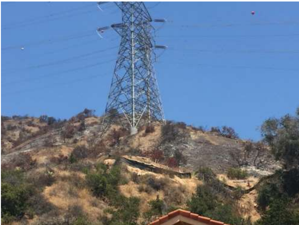
Figure 2: Tower M27-T3 after the recent fire in Duarte, Segment 7.
