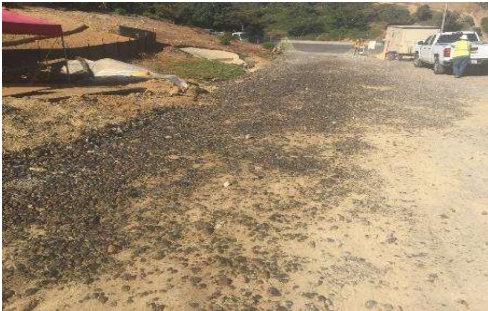
Figure 5: Large hydraulic spill from the HDD rig at VC #11, 500 kV Underground.
