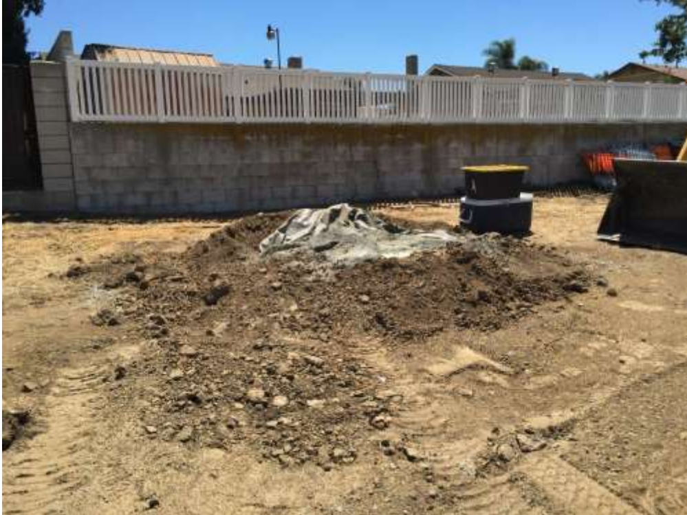
Figure 1: SCE monitors observed inadequate concrete washout containment near VC #12 on August 15. Photo courtesy of SCE.
