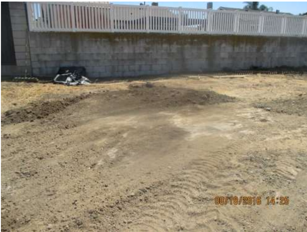
Figure 2: SCE directed crews to remove the inadequate concrete wash out. Photo courtesy of SCE.
