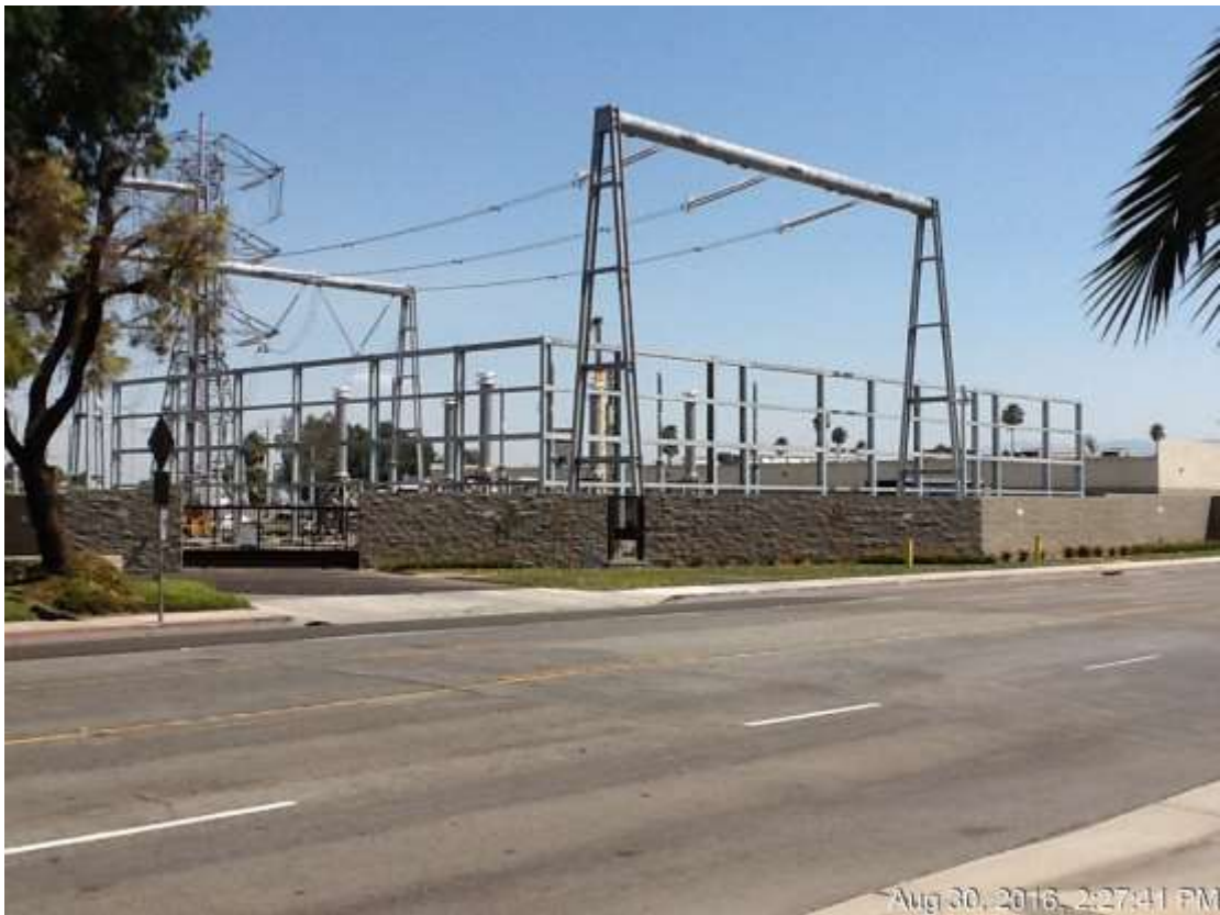
Figure 4: Barrier screen supports at the ETS, 500 kV Underground, Screen installation will occur in the next few weeks.
