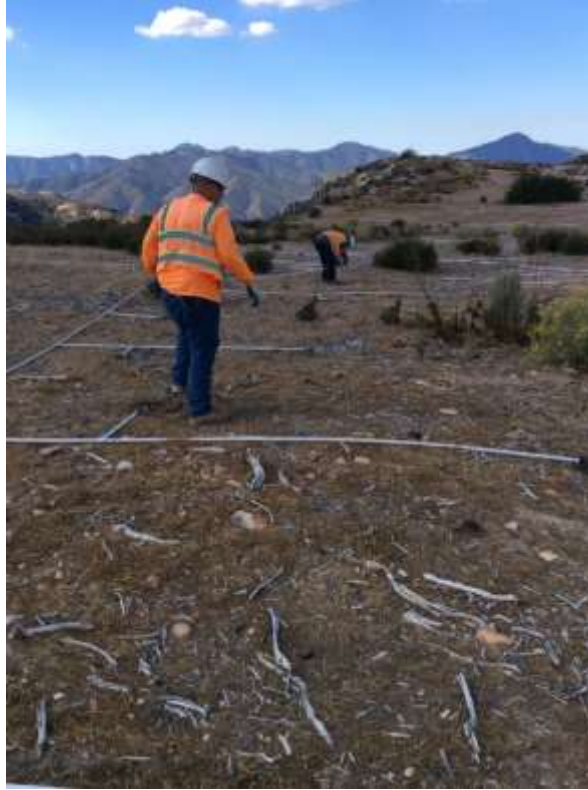
Figure 1: Irrigation installation and testing at Chileao Helicopter Assembly Yard, Segment 6. (Photo courtesy of SCE.)
