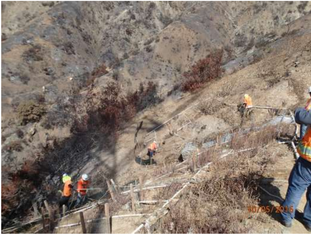
Figure 3: BMP repairs at Tower M27-T2 near Duarte, Segment 7. (Photo courtesy of SCE.)
