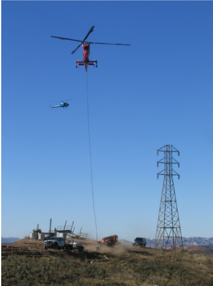
Figure 1: Helicopter use in Section 2 on the ANF for equipment mobilization to micropile sites.
