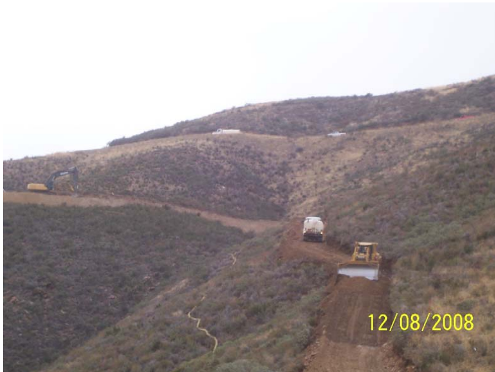
Figure 2: Building of Spur Road 41 with erosion control measures (straw wattles and rip rap).
