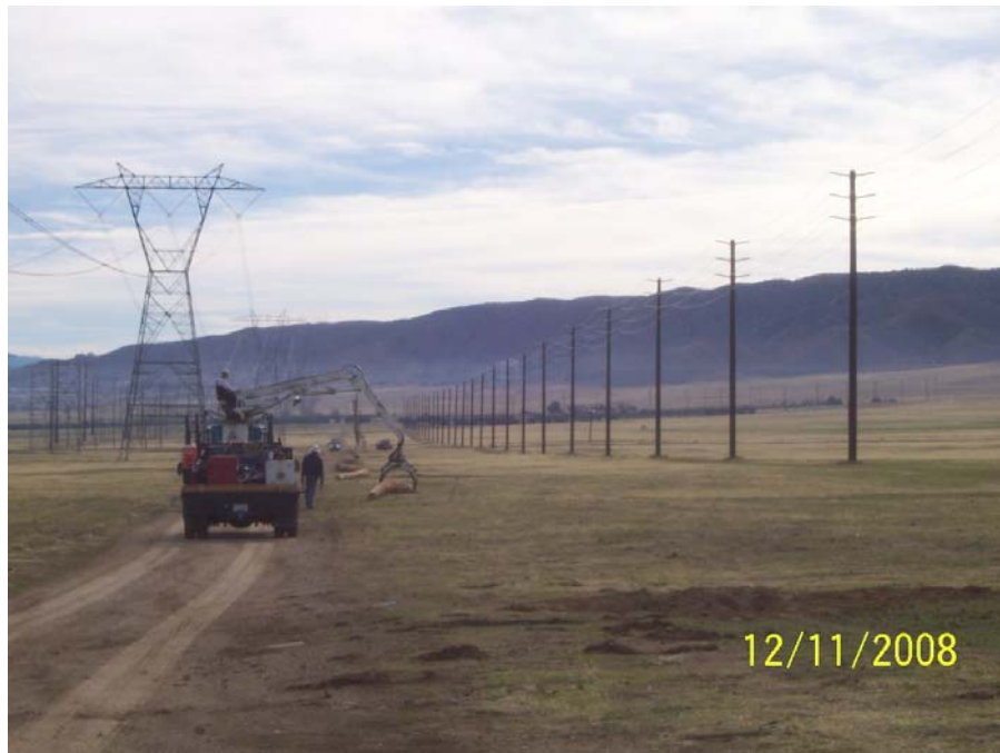
Figure 3: Realignment of the existing 66 kV line to accommodate the new 500 kV towers.
