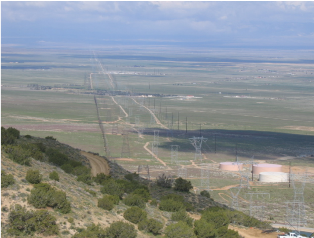
Figure 5: View of the Segment 2 right-of-way looking towards the Antelope Substation. On the left is the newly relocated 66 kV wood pole line with the partially assembled new 500 kV towers to their immediate right.
