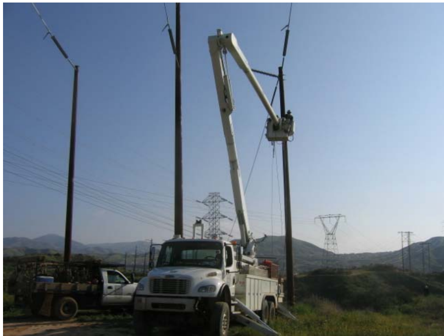
Figure 2: Crews preparing to remove the conductor from the Shoofly line in Santa Clarita.
