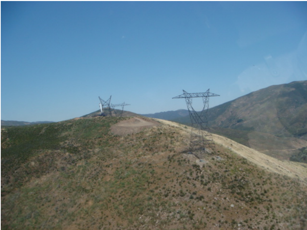
Figure 2: Tower assembly on the ANF. Note the disturbance area at the first tower (helicopter construction) and at the second tower (conventional construction).
