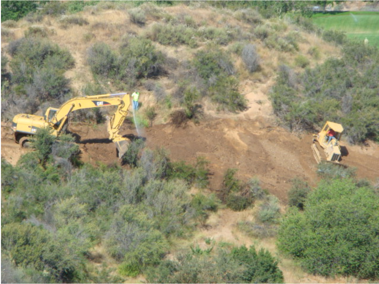
Figure 1: Shoofly road re-compacting at SF 4 in Section 1. Revegetation is planned for later this year.
