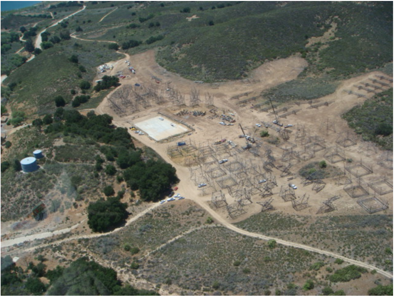
Figure 3: Tower section assembly at the Hydrant Yard to be flown into place with the Sky Crane.
