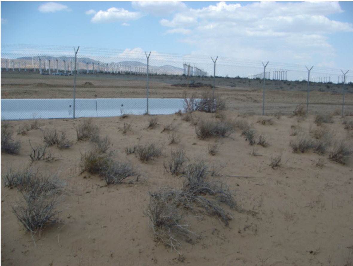
Figure 5: K-rail installed along the tortoise fencing surrounding the Windhub Substation site to protect off-site sand drifts in the area of the tortoise burrow.
