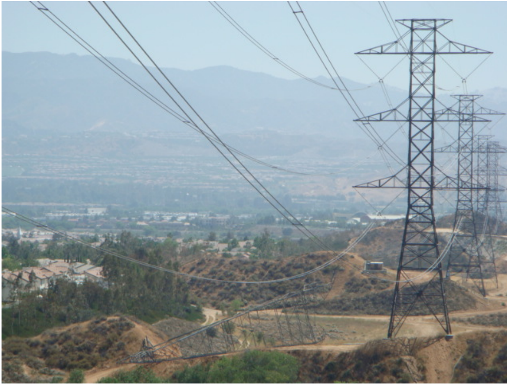
Figure 1: Wreck-out of the 220 kV structures near Tower 5 by SCE and UPC crews, Segment 1, Section 1.
