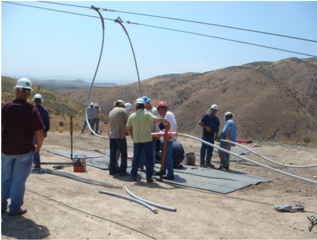
Figure 2: Wire splicing using implosive sleeves near Tower 33 in the ANF, Segment 1, Section 2.
