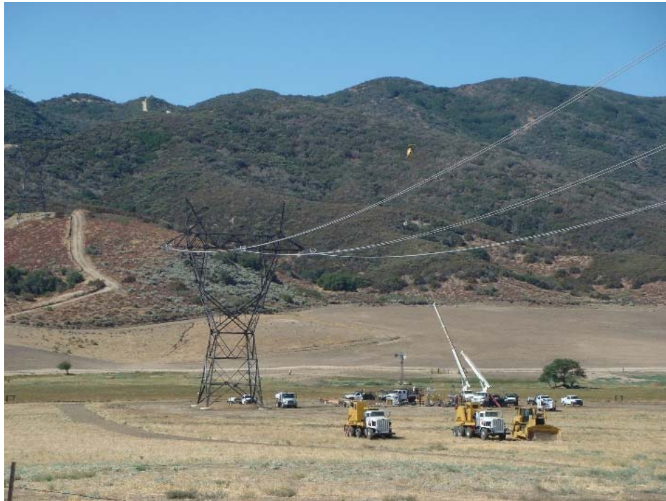
Figure 2: Conductor installation between Towers 84 and 92, the last portion of the project on the ANF requiring stringing.
