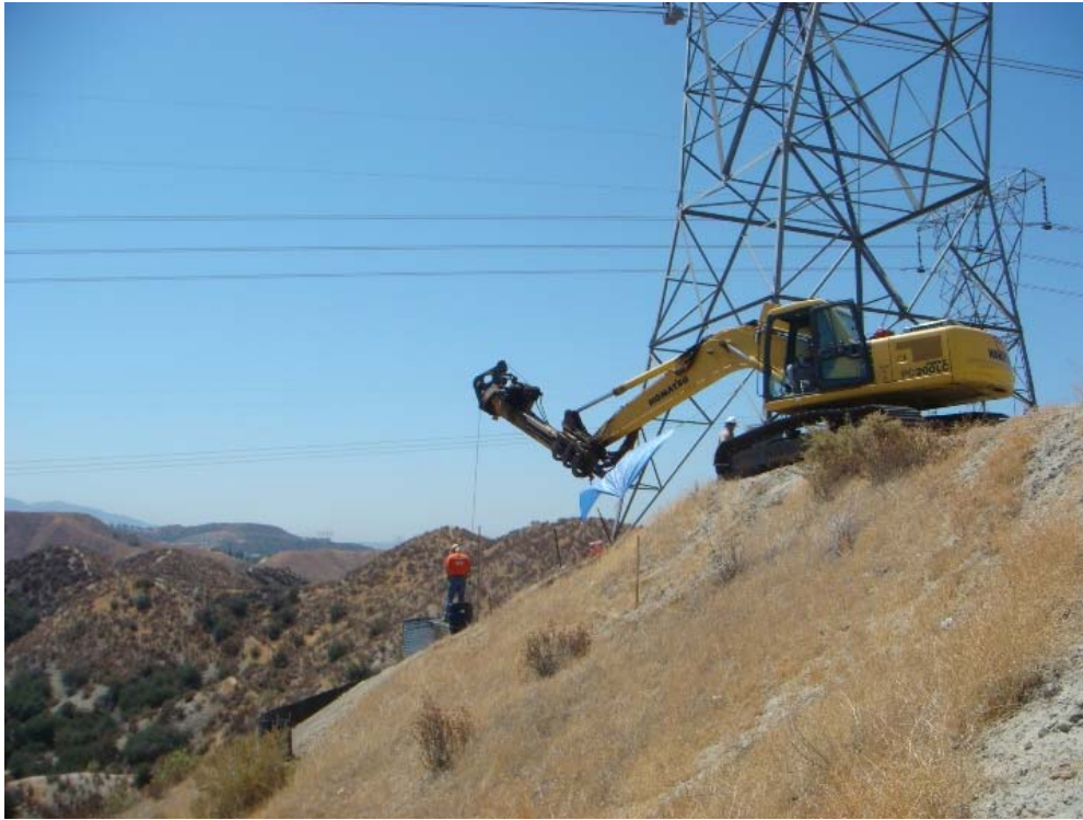
Figure 1: Hand excavation of new tower foundations at existing Tower M24T-1 required for its modification, Segment 1, Section 1.
