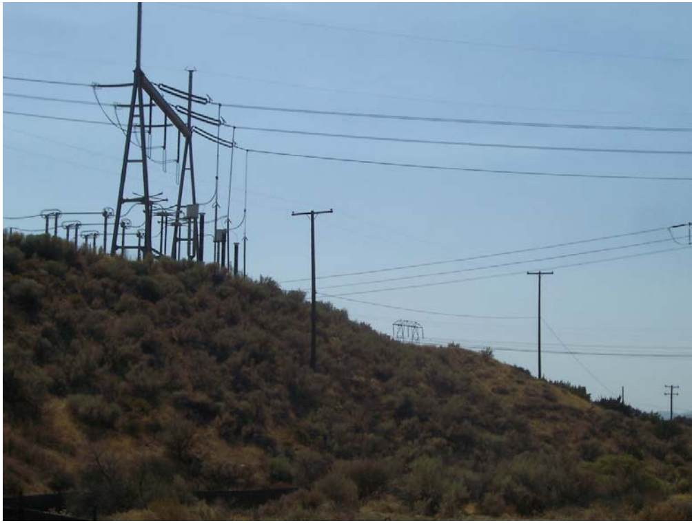
Figure 4: Location of the 12 kV Distribution Line Bootlegger Segment 2.
