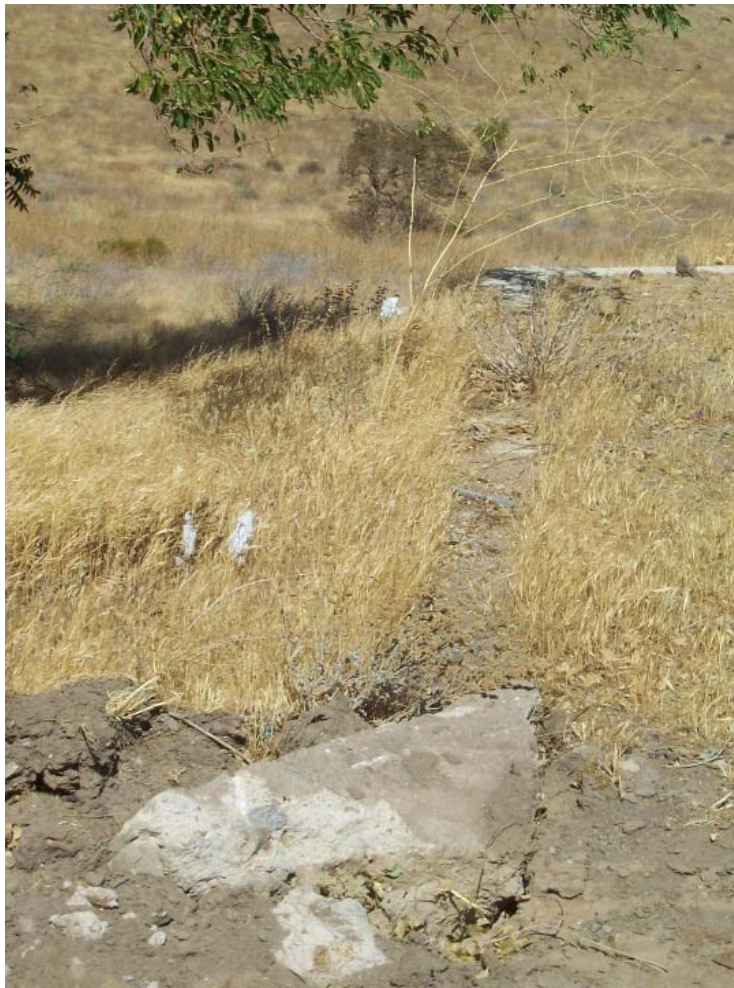
Figure 2: Damage to a historic foundation feature in Section 3.
