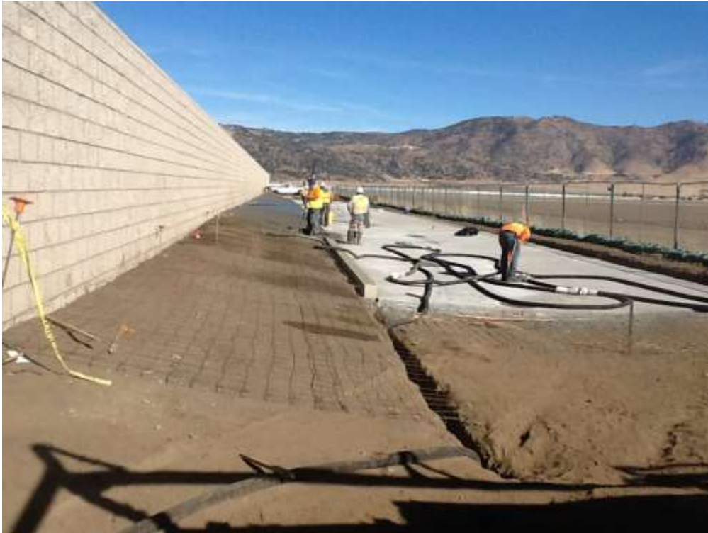
Figure 1 – Professional Construction crews graded and poured the concrete v-ditch surrounding the Banducci Substation site.
