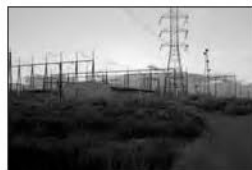
Lugo Substation Garage
