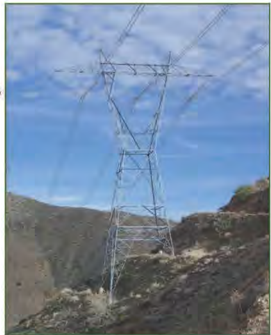
High voltage (500-kV) AC transmission lines
