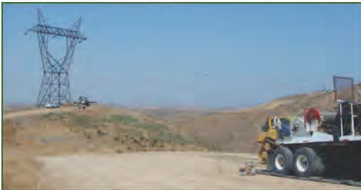
Pulling phase of a wire-stringing operation. Note the reel of conductor on the right side of the photo.
