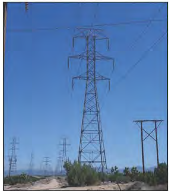
Example of a 220-kV double-circuit LST.
