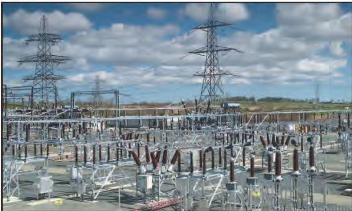
Electric substation, with transformers and associated equipment shown in the foreground, and transmission towers and lines present in the background. (photo credit: www.ethospower.in )
