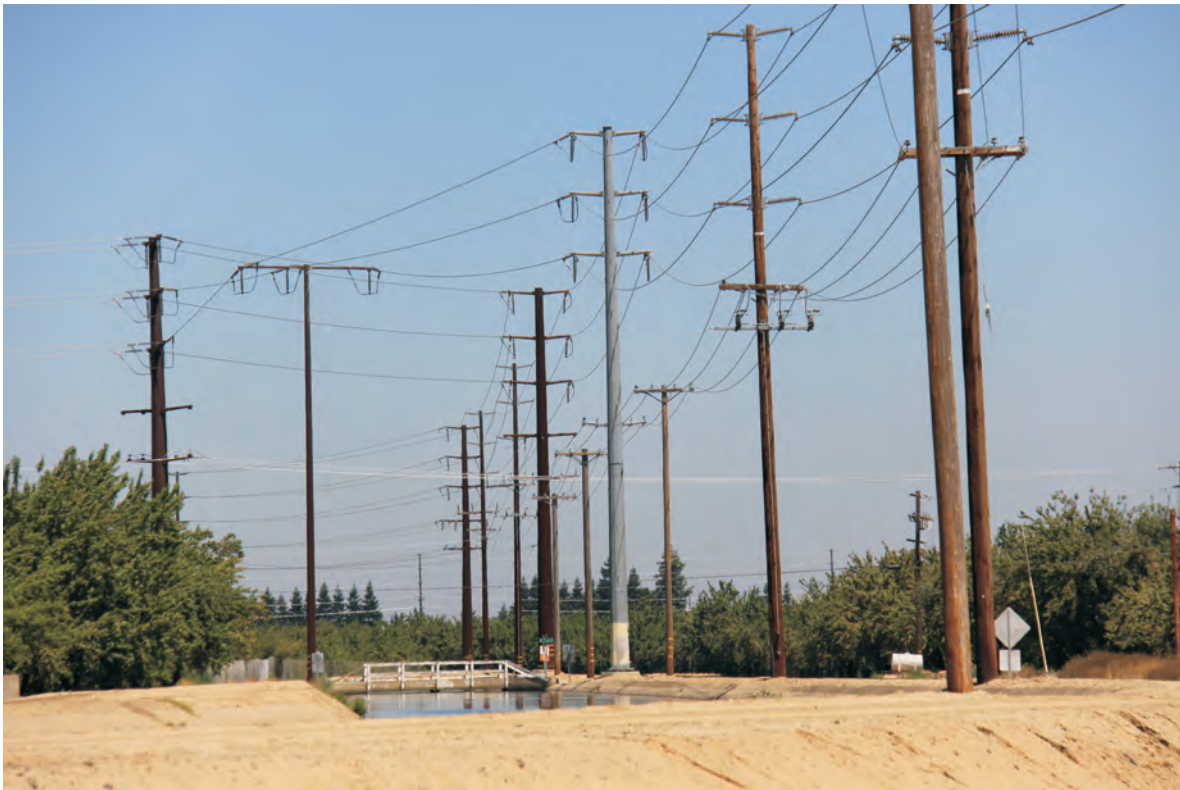
Photograph 16. Group of TSPs, LDS poles, and wood poles along Canal Avenue.
