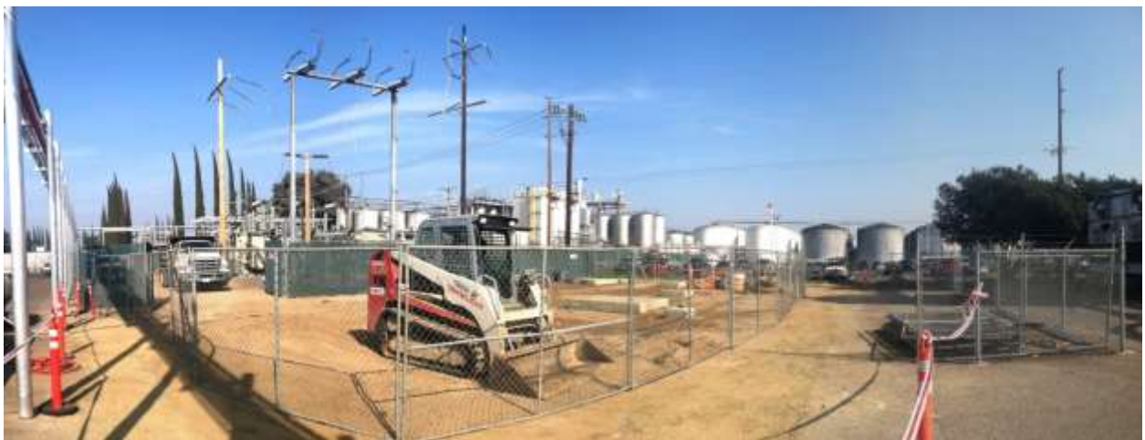
Figure 3 – Construction continued at the Gallo Substation during the subject period. View northeast from southwest corner of future substation area, 01/20/15 top, 01/29/15 middle, 02/03/15 bottom.
