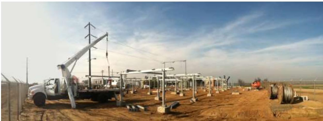
Figure 1 – Structure installation occurred at the Cressey Substation during the subject period. View from southeast corner of substation facing northwest, 01/08/15 top 01/20/15 middle, 02/03/15 bottom.
