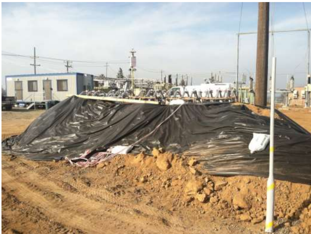
Figure 4 – Soil pile containment is in place at the Cressey Substation work area. View northwest, 02/03/15.
