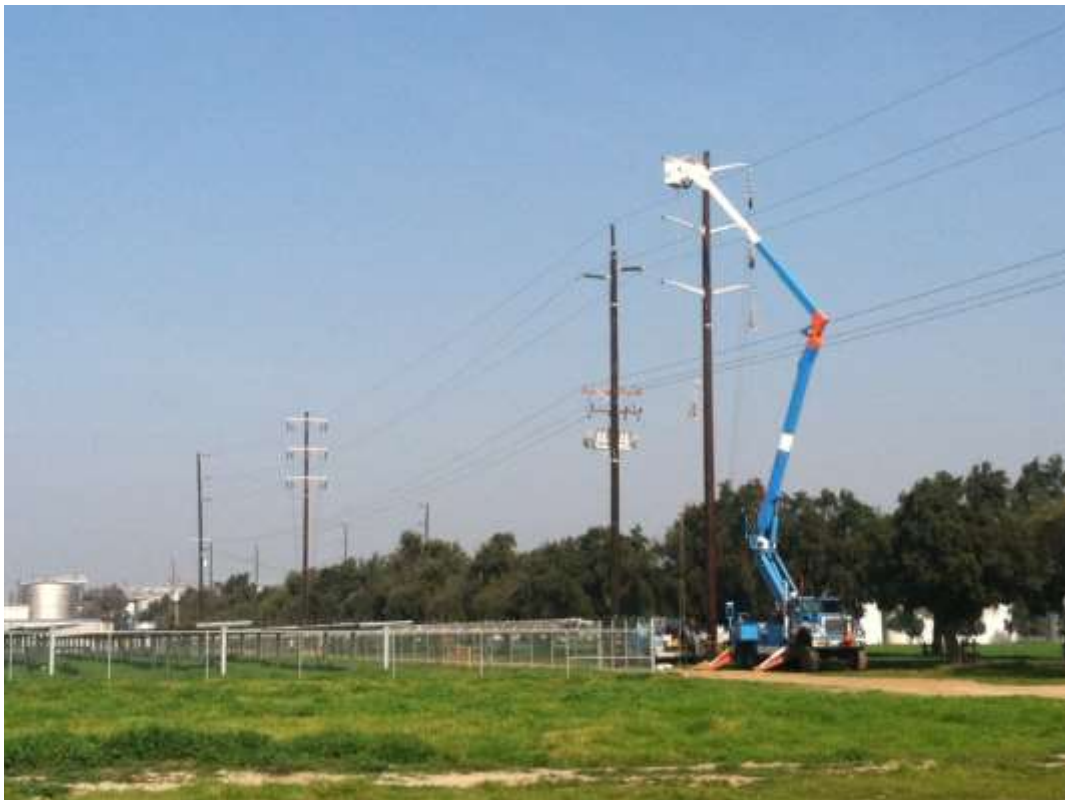
Figure 3 – Installation of conductor along recently installed transmission poles occurred adjacent to the temporary Shoo Fly poles. View northeast, 02/03/15.
