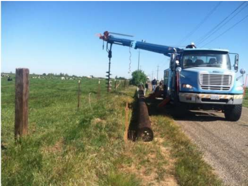
Figure 6 –Crews install a pole between elderberry bush buffers along West Lane. View north. (Photo provided by PG&E)
