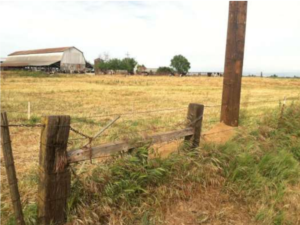
Figure 3 – The pole pictured here was adjusted to avoid a seasonal ponded area along Palm Avenue. Resource buffer delineators were in place during installation. View northeast, 04/01/15.
