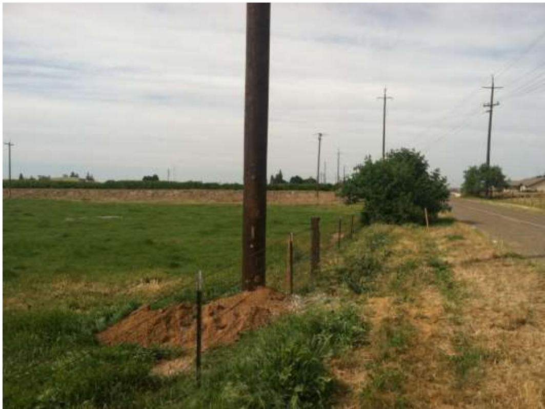
Figure 5 –A wood pole is seen installed adjacent to an elderberry bush buffer along West Lane. View northwest, 03/25/15 above, 04/01/15 below.
