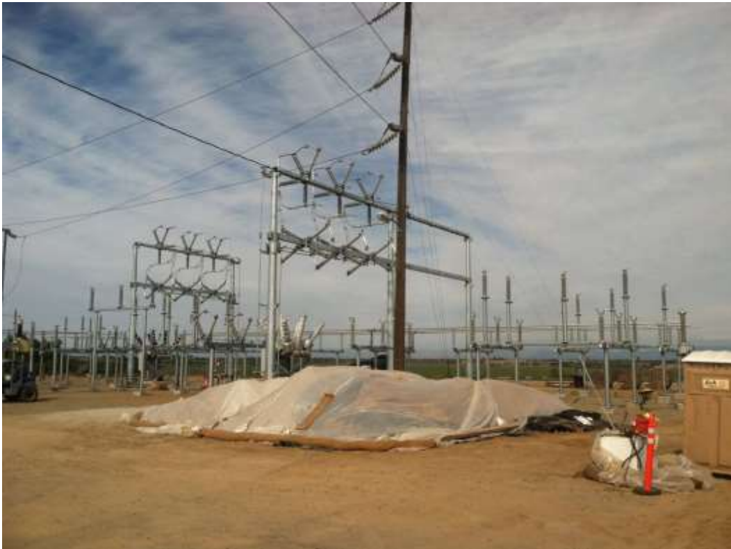
Figure 2 – Erosion control devices continue to be maintained. View northeast, 04/01/15.
