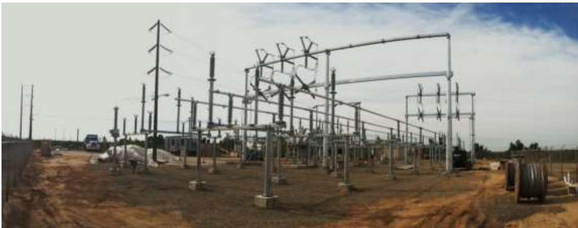
Figure 1 – Structure installation continued at the Cressey Substation during the subject period. View from southeast corner of substation facing northwest, 01/08/15 above 3/19/15 middle, 4/01/15 below.
