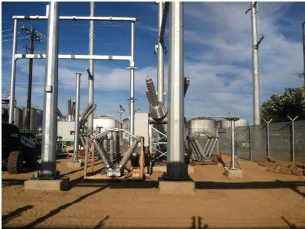
Figure 2 – Structure installation continued at Gallo Substation during the subject period. View east, 5/29/15.
