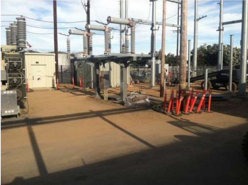
Figure 1 – Structure installation continued at the Gallo Substation during the subject period. View southeast, 5/29/15.
