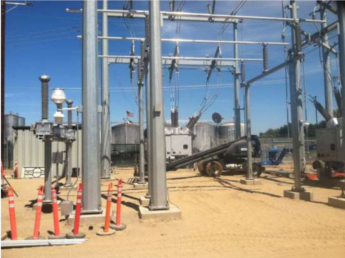
Figure 1 – Structure installation continued at the Gallo Substation during the subject period. View east, 6/19/15.
