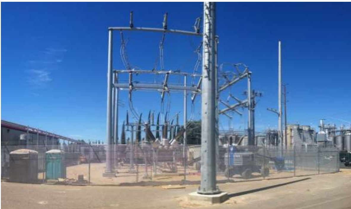
Figure 2 – Crews continued installing structures at the Gallo Substation during the subject period. View north, 6/19/15.
