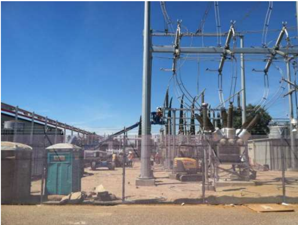
Figure 2 – Crews continued installing structures at the Gallo Substation during the subject period. View north, 6/30/15.
