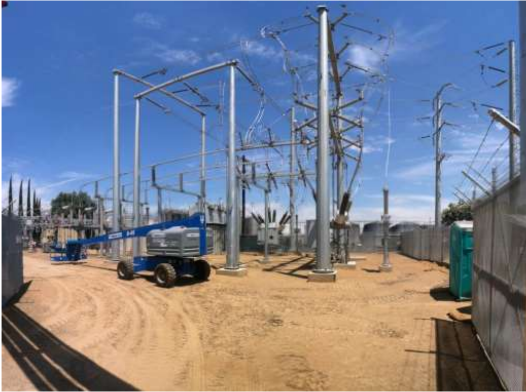
Figure 1 – Construction work continued at the Gallo Substation during the subject period. View northeast, 7/2/15.
