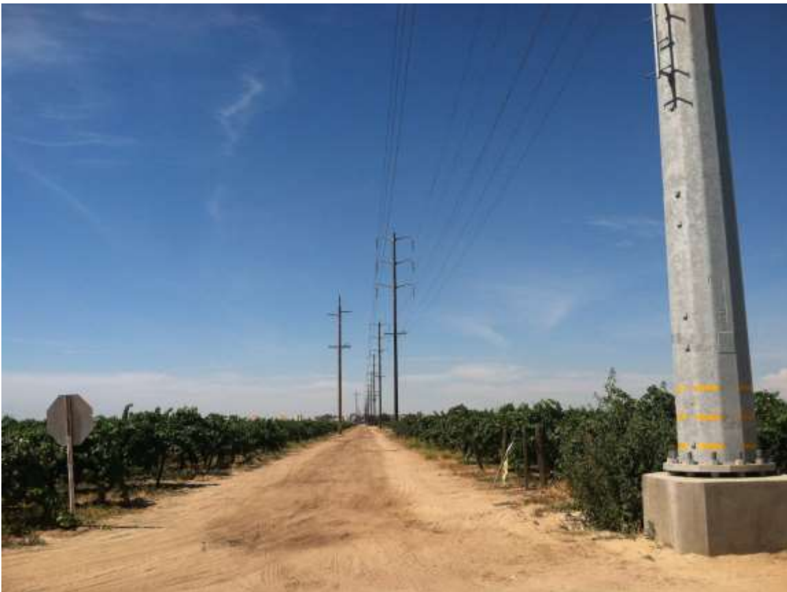
Figure 3 – Removal of the Shoo-Fly (left row of poles and line) occurred during the subject period. View
