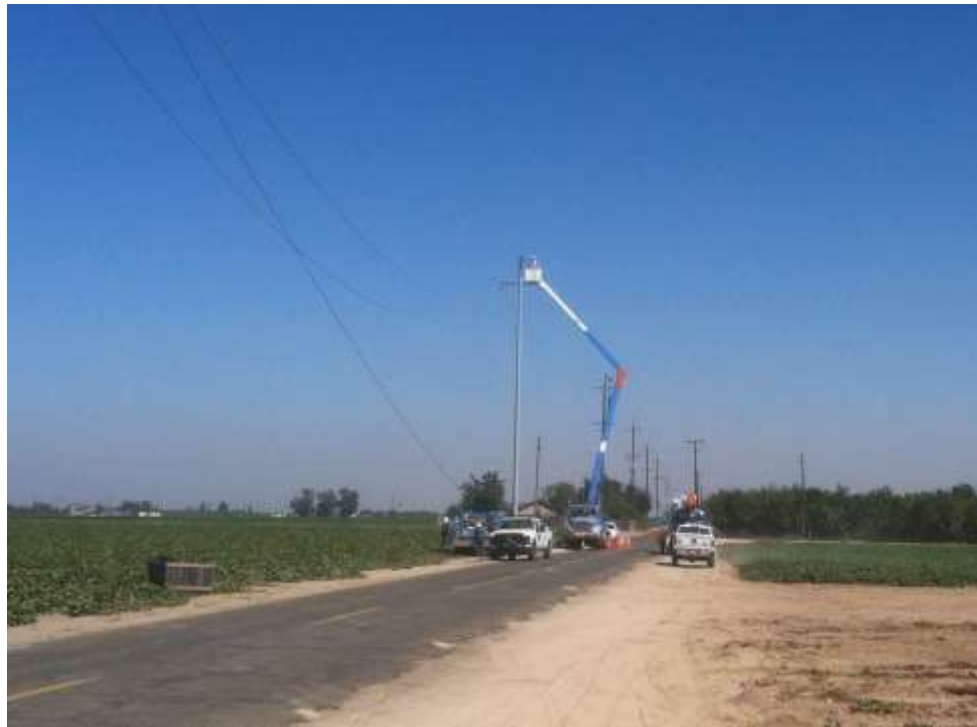
Figure 2 – Crews installed conductor along Magnolia Avenue during the subject period. View east 9/9/15.
