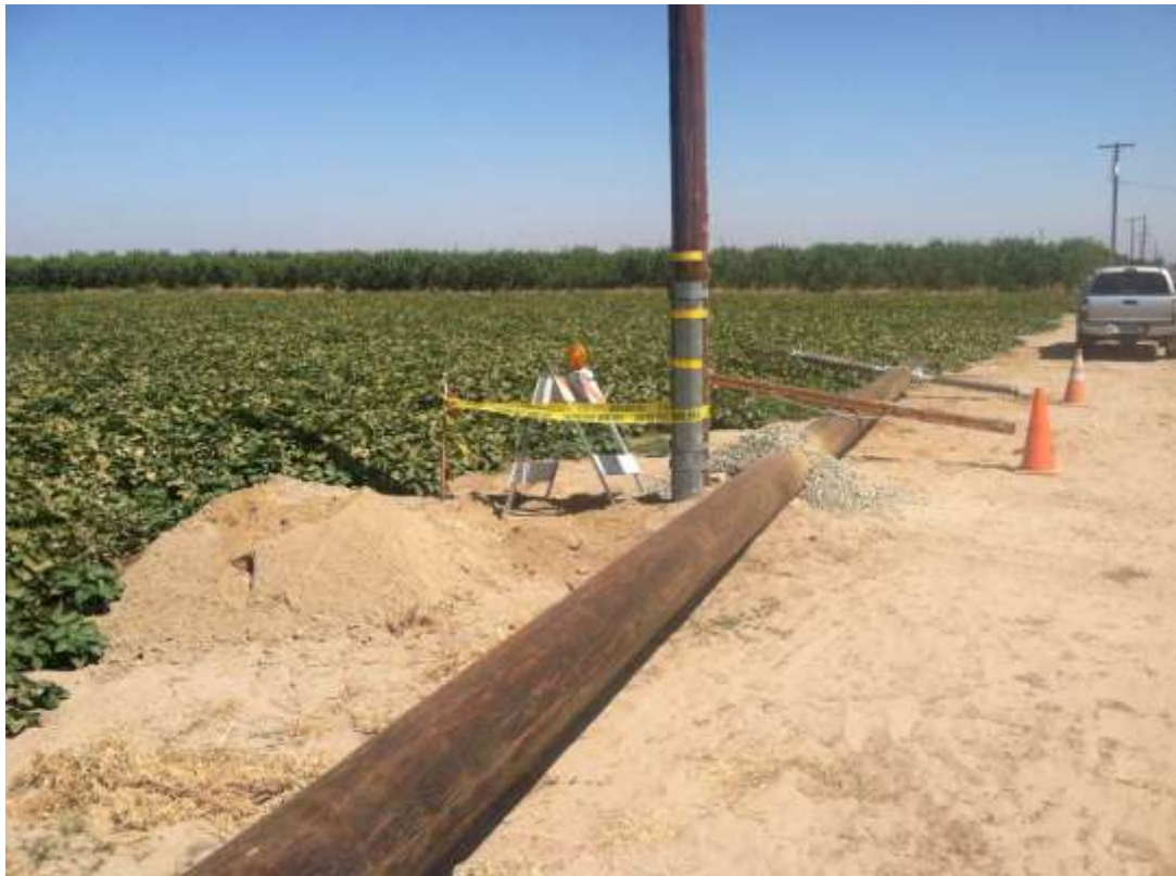
Figure 4 – Augered holes along Magnolia Avenue were securely covered and clearly marked during the subject period. View east 9/9/15.
