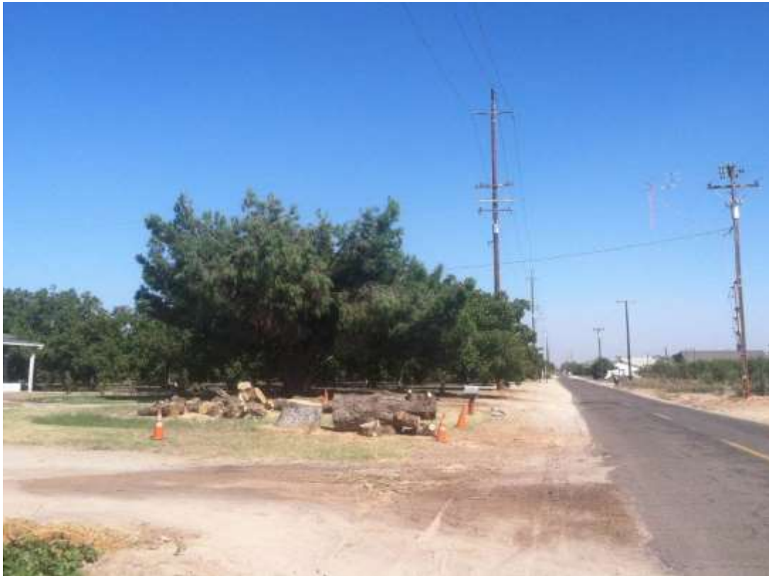
Figure 3 – Tree removal work was completed along Magnolia Avenue during the subject period. View east 9/9/15.
