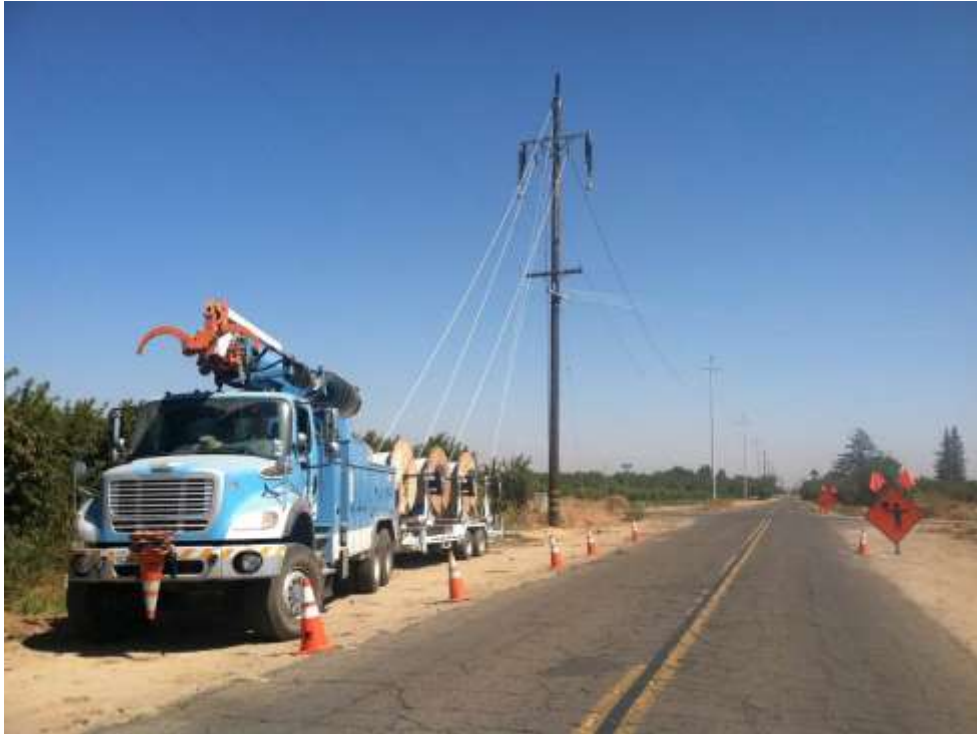
Figure 1 – Crews installed conductor along Magnolia Avenue during the subject period. View east 9/9/15.
