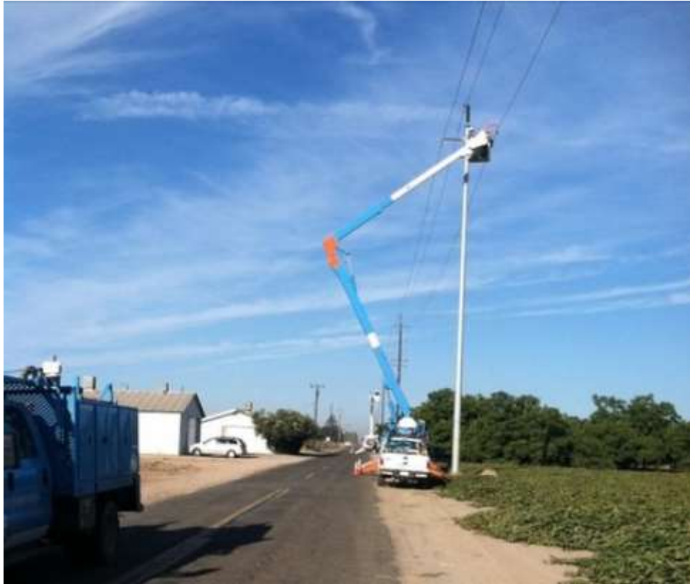
Figure 1 – Crews installed conductor along Magnolia Avenue during the subject period. View west 9/25/15 (photo provided by PG&E).
