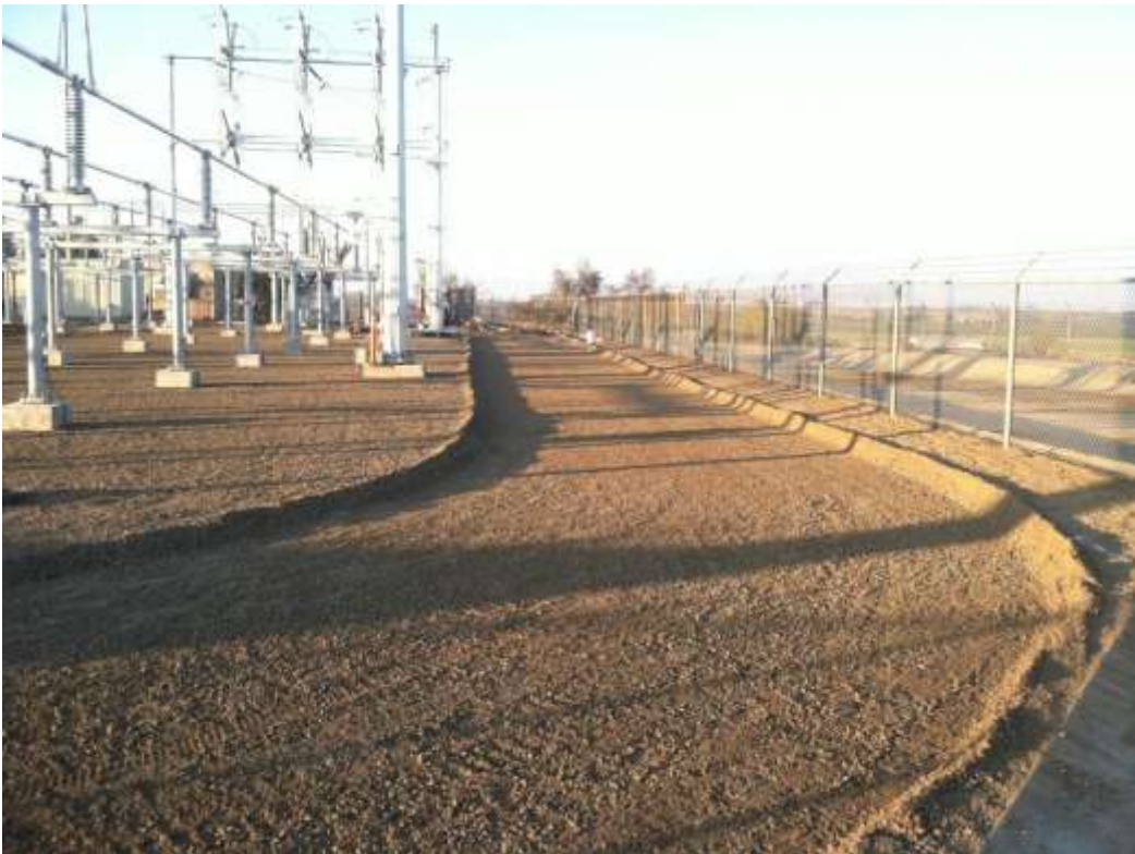
Figure 2 – Grading and paving preparation occurred at Cressey Substation during the subject period. View north 11/19/15.
