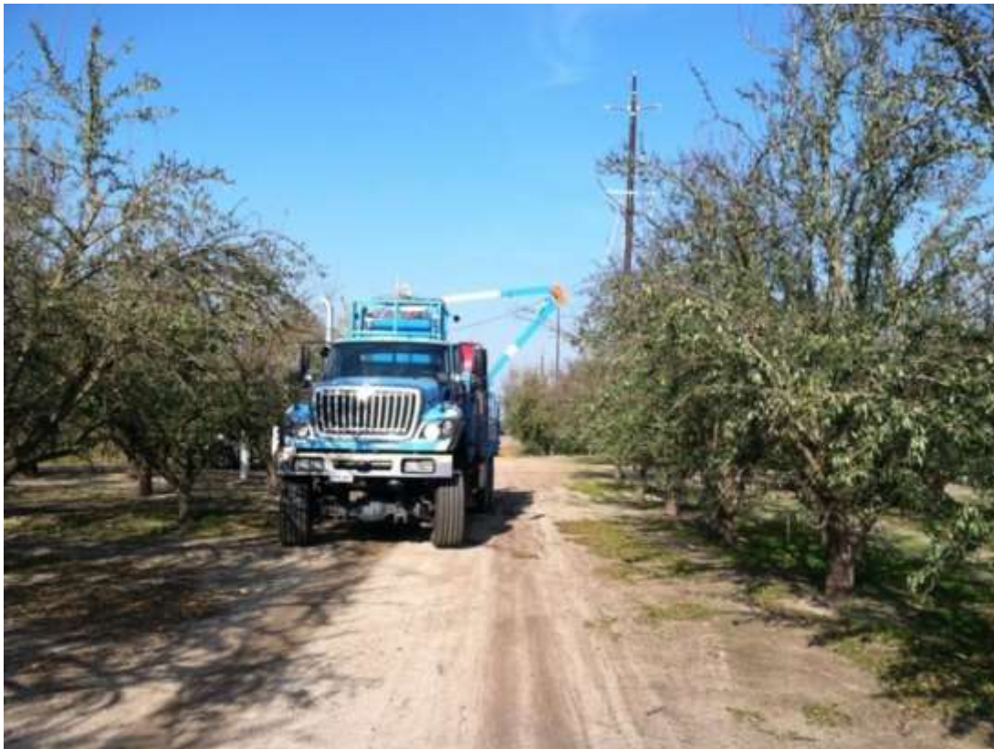
Figure 4 – Line work continued during the subject period. View north along Arena Way (Photo provided by PG&E).
