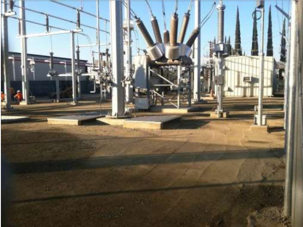
Figure 1 – Grading and paving activities continued at Gallo Substation during the subject period. View northwest, 11/19/15.
