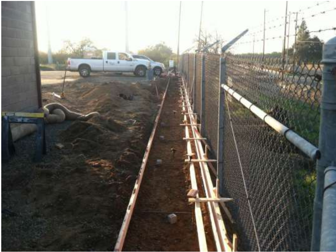
Figure 3 – Culvert installation continued at Cressey Substation during the subject period. View west, 11/19/15.
