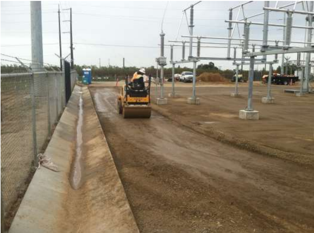
Figure 3 – Grading and paving work continued at Cressey Substation during the subject period. View west, 11/24/15.
