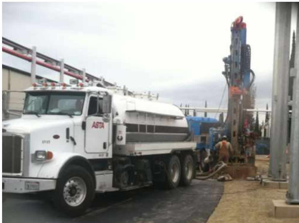
Figure 2 – Drilling for grounding wells occurred at the Gallo Substation during the subject period. View north 11/24/15.
