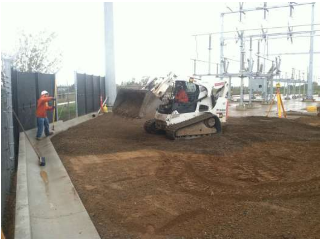
Figure 4 – Grading and paving work continued at Cressey Substation during the subject period. View southeast, 11/24/15.
