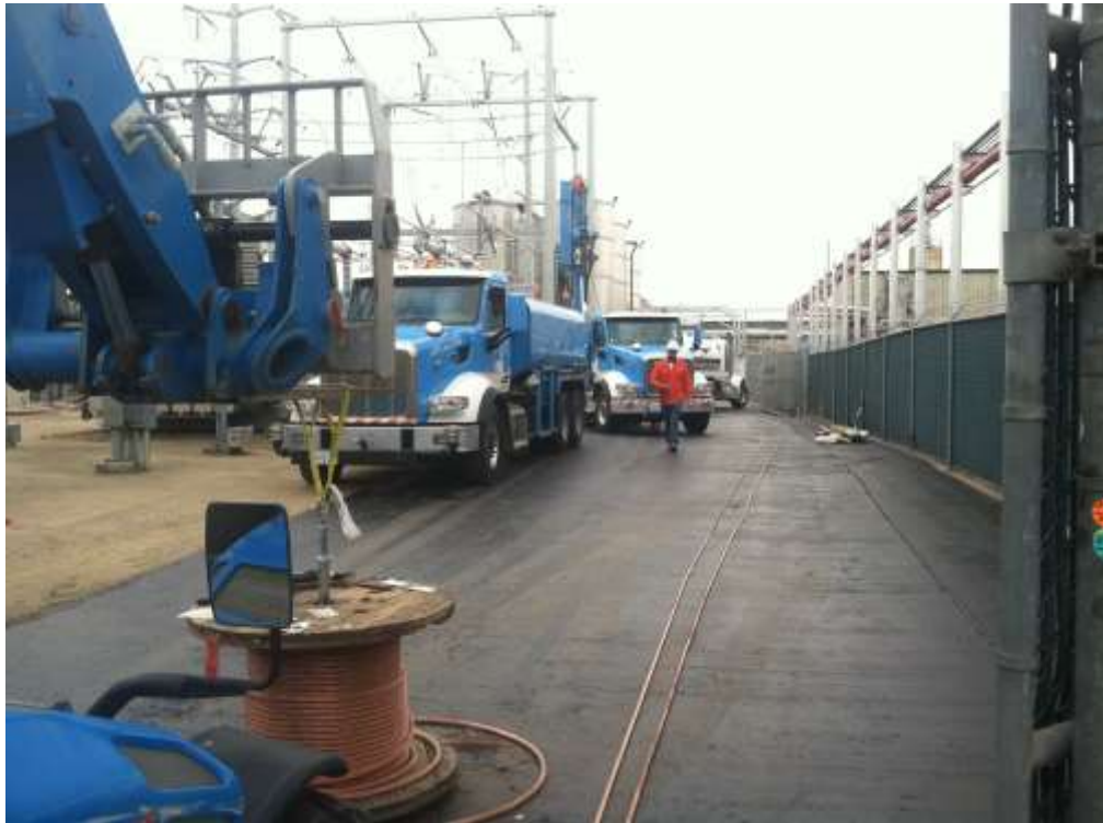
Figure 1 – Paving activities were complete at Gallo Substation during the subject period. View south, 11/24/15.
